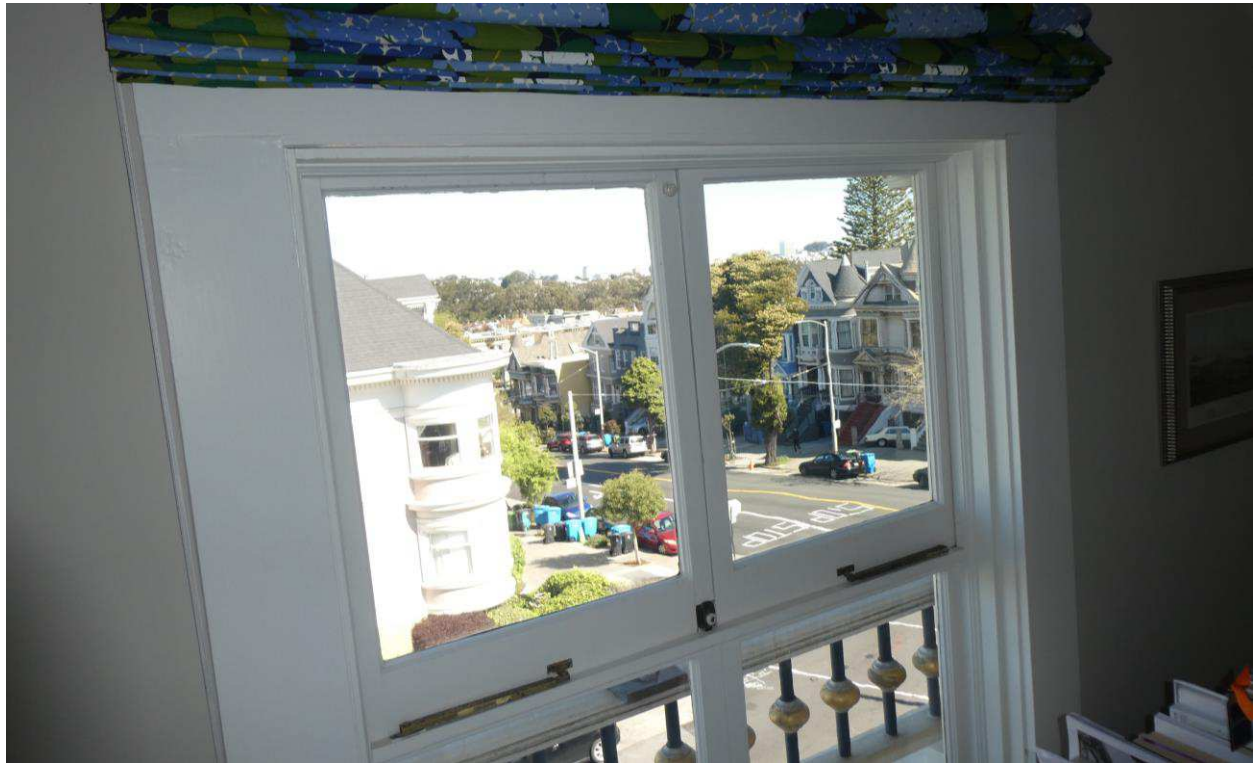
Figure 39: Interior detail of the attic window at the Waller Street gable end, upper casement sash.
