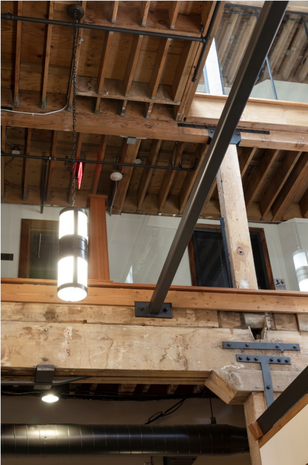
Figure 26: Wood support pillar from ground to third floor, 2019. Looking west. Courtesy of Henrik Kam.
