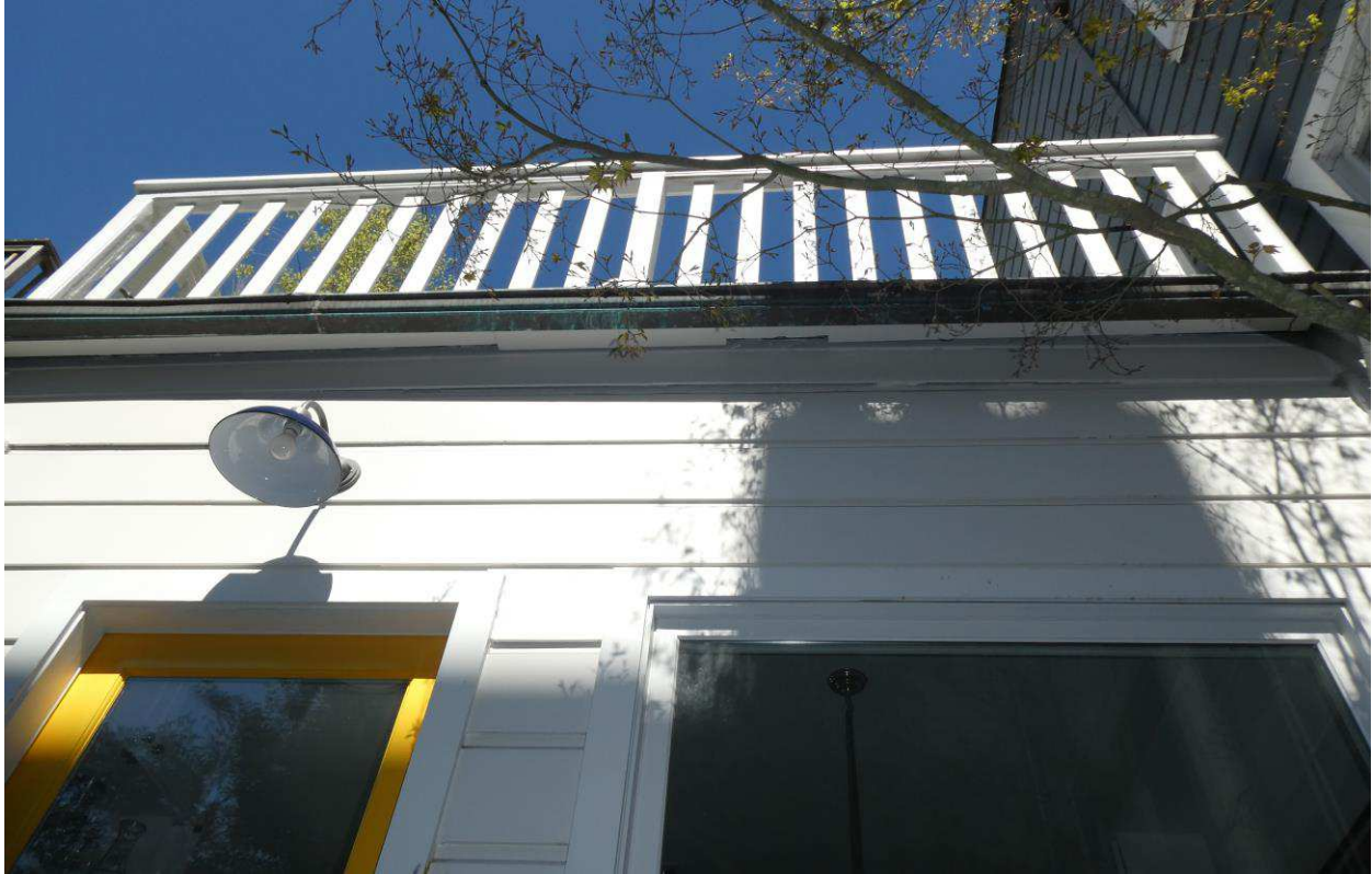
Figure 43: Detail of the bulging top siding board at the southeast side of the first floor kitchen.
