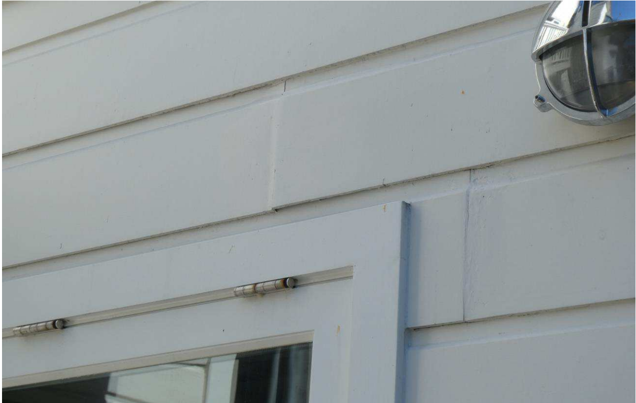
Figure 44: Detail of bulging siding at the upper corner of the window, southwest side of the first floor kitchen. Note bulging at the lower corner in (Figure 45).
