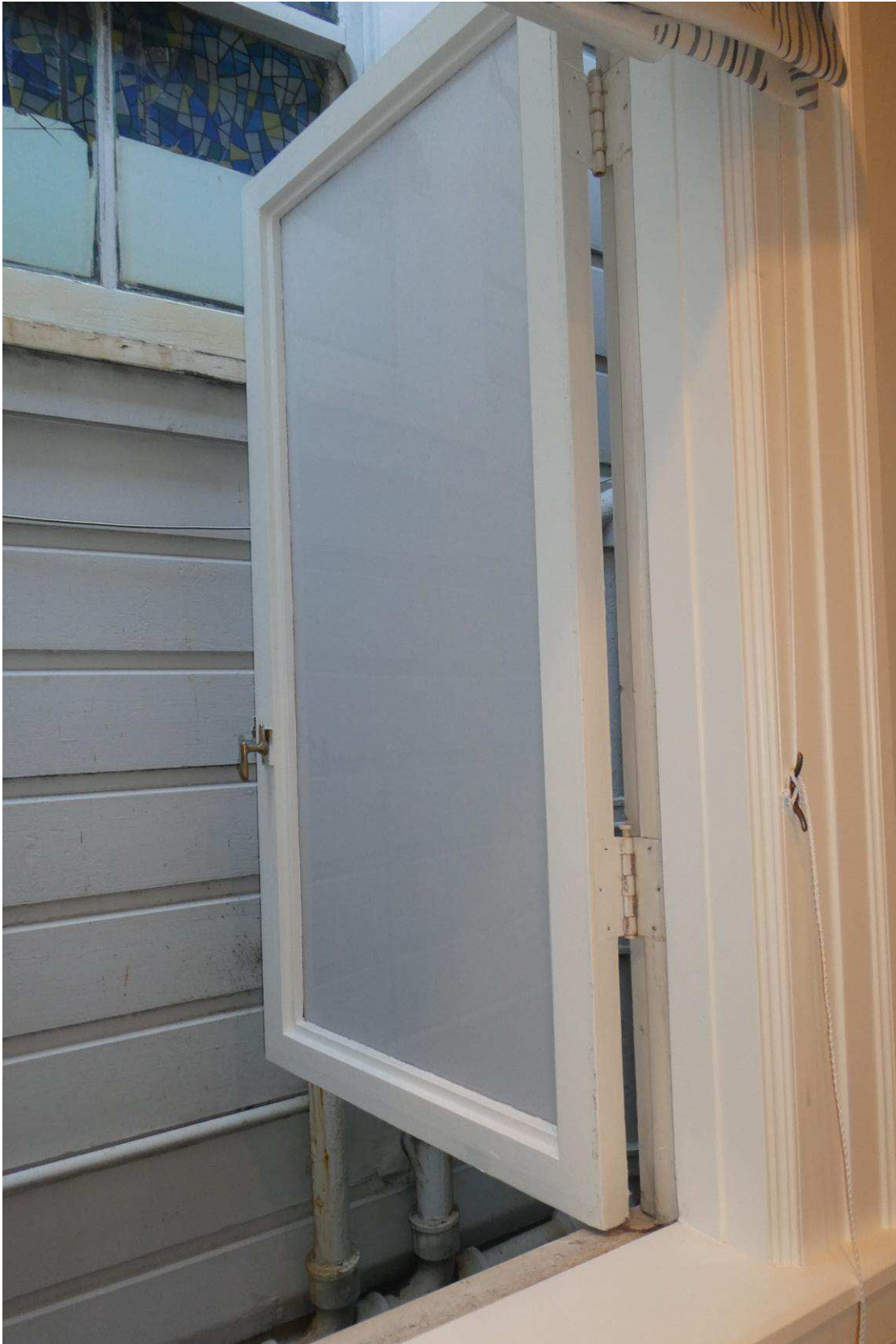
Figure 49: Non-historic casement sash at the second floor looking into the northeast lightwell.
