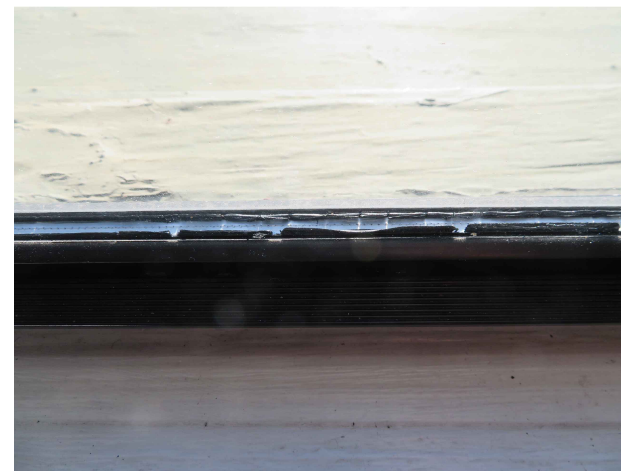
8 DETERIORATED GASKET PC: ARG
