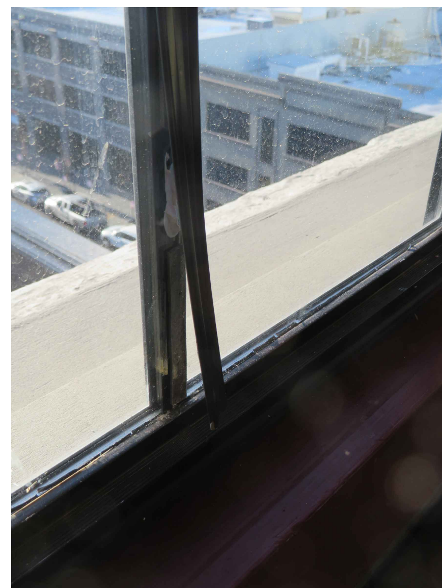
7 ADHESIVE FAILURE AT MUNTIN PC: ARG
