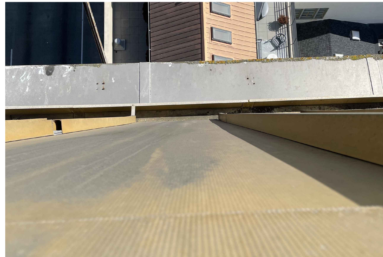
4 WEATHERED FINISH AND DISPLACED BATTENS PC: ARG/CS
