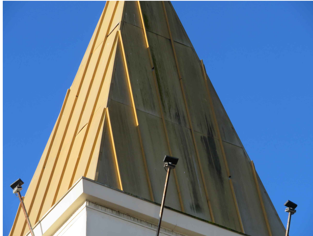
1 GEN. SOILING, WEATHERED FINISH, DISP. BATTENS PC: ARG
