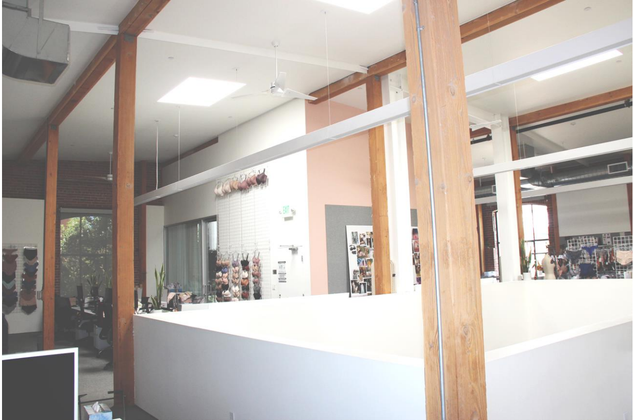
Figure 44. Heavy timber framing on the third floor; view toward northwest. Note moment frame at right.
