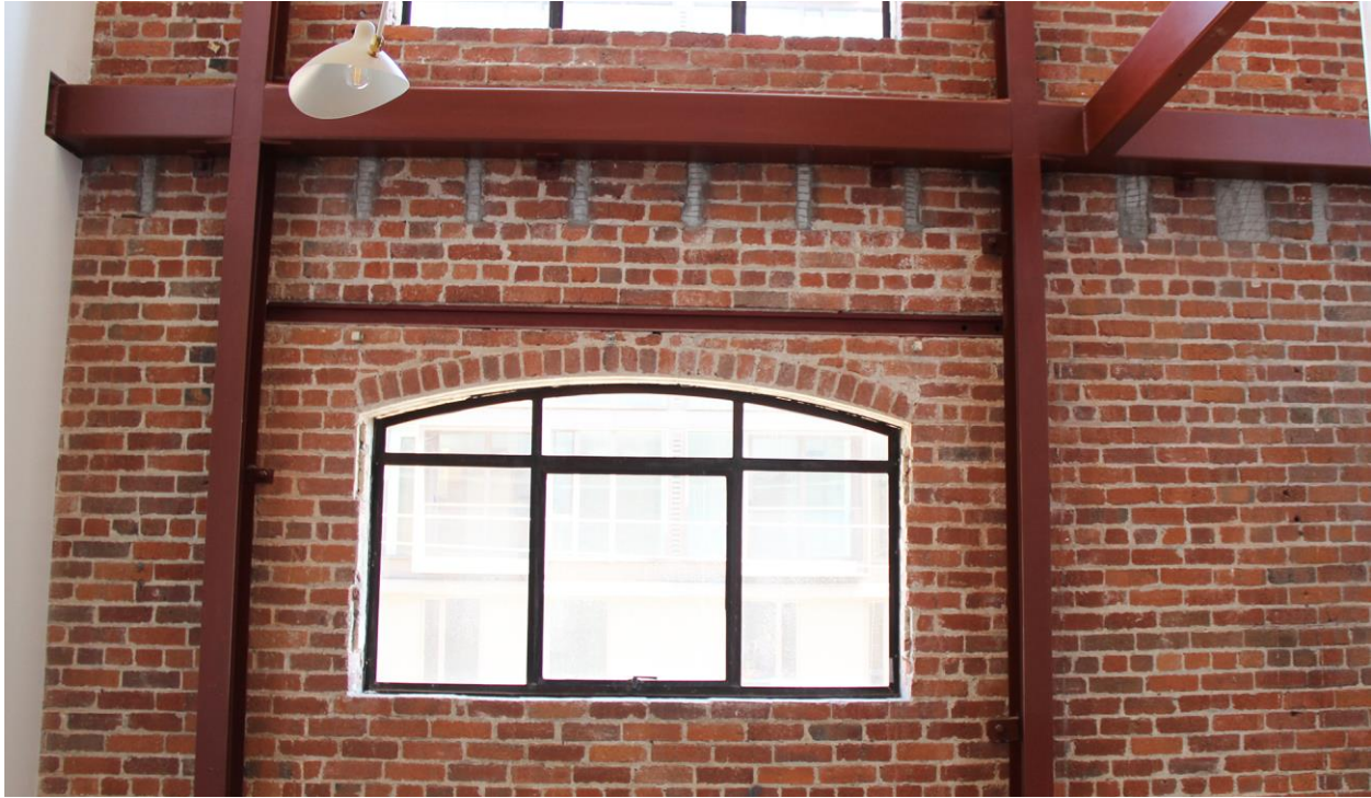
Figure 42. Interior brick at the second-floor level above the lobby on 19 th Street. Note the filled joist pockets.
