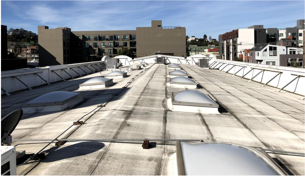
Figure 25. Detail of roof showing parapet braces and rolled roofing materials; view toward west.
