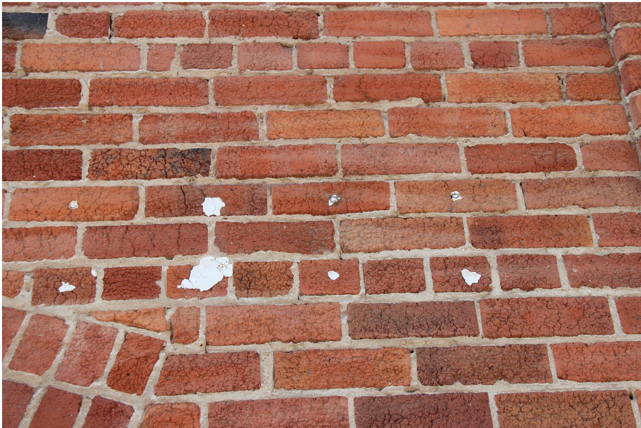
Figure 12. detail of brick facing 19 th Street. Note old paint residue and cracked and missing mortar.
