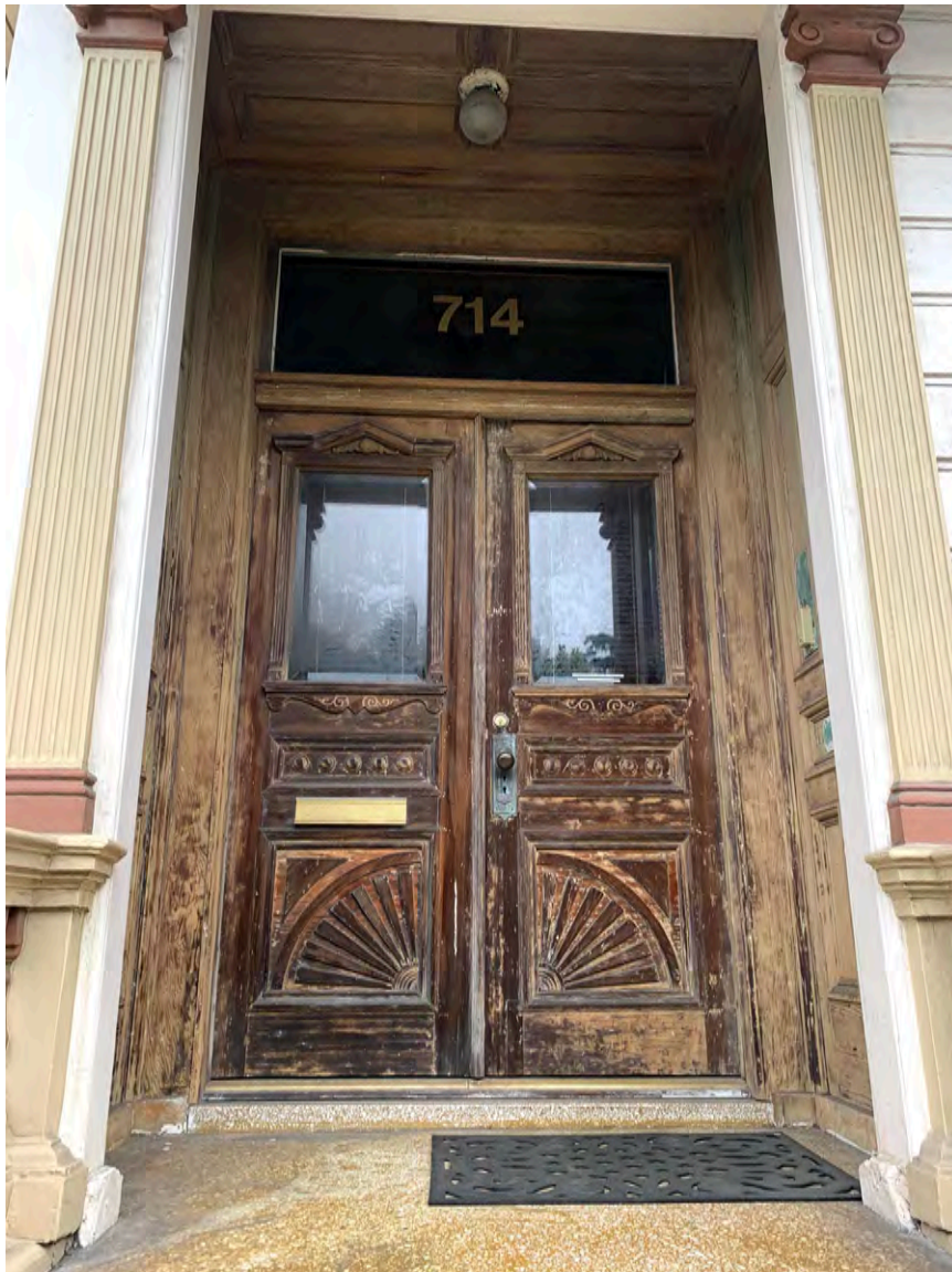
Photograph 9: 714 Steiner, primary Steiner Street façade, detail of entry landing and front door.
