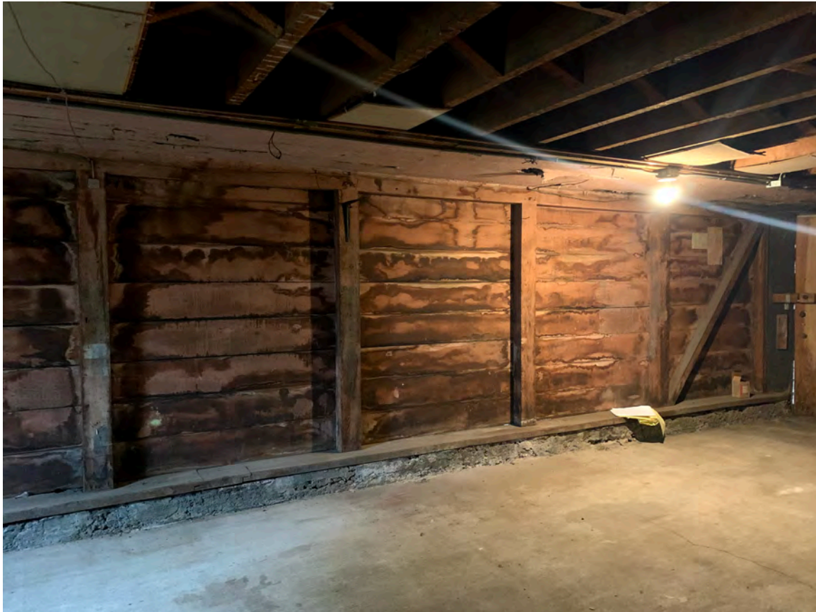
Photograph 52: South wall conditions in garage showing water damage
