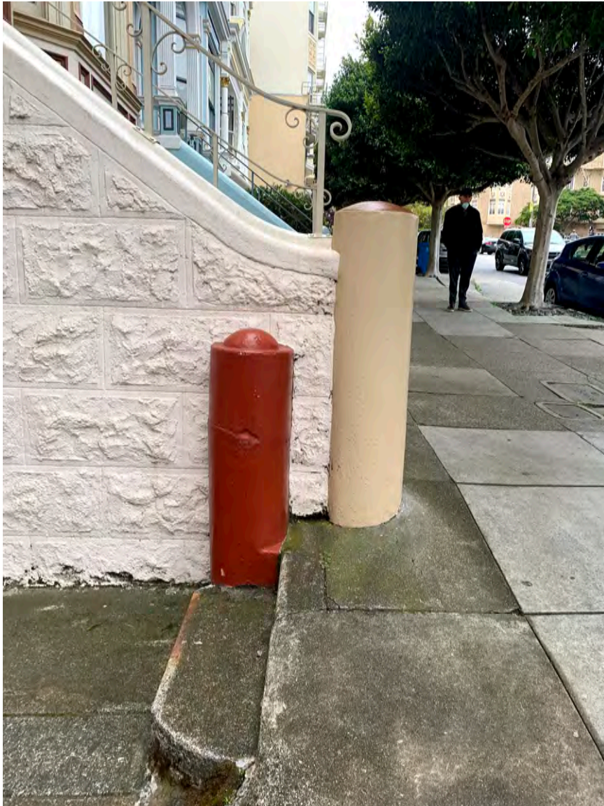
Photograph 13: 714 Steiner, primary Steiner Street façade, detail of stair bollards and “rusticated” concrete pattern on stairs.
