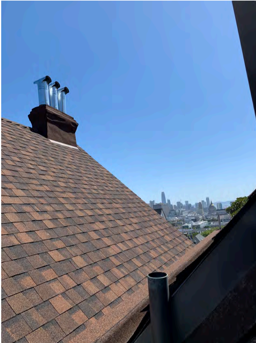
Photograph 34: Detail of roof near light well showing chimney covering and roofing composition shingles, looking east toward City Hall.
