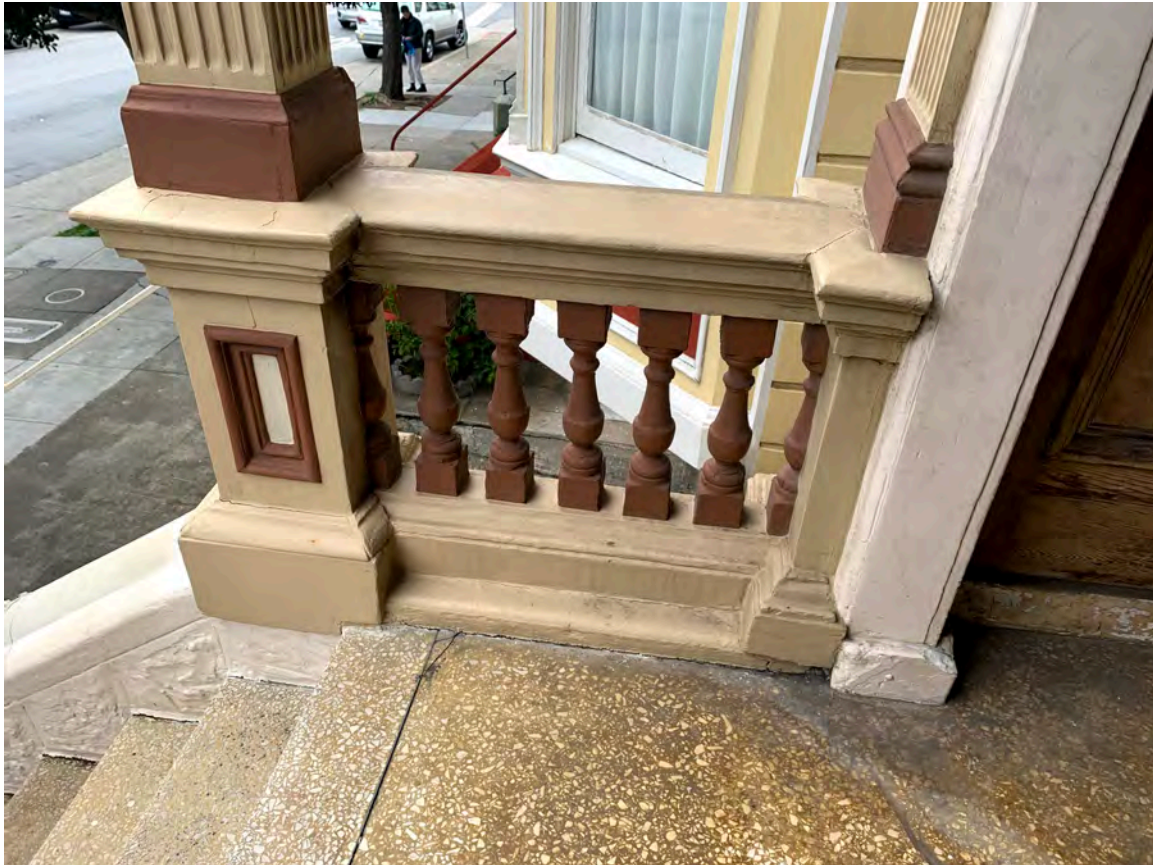
Photograph 16: 714 Steiner, primary Steiner Street façade, detail of porch terrazzo condition and past intervention at porch
