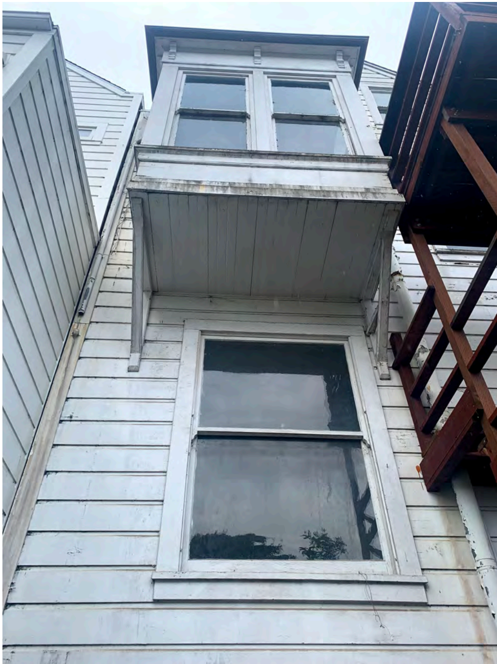
Photograph 28: Detail of rear, east façade, upper level with boxed bay window and supports
