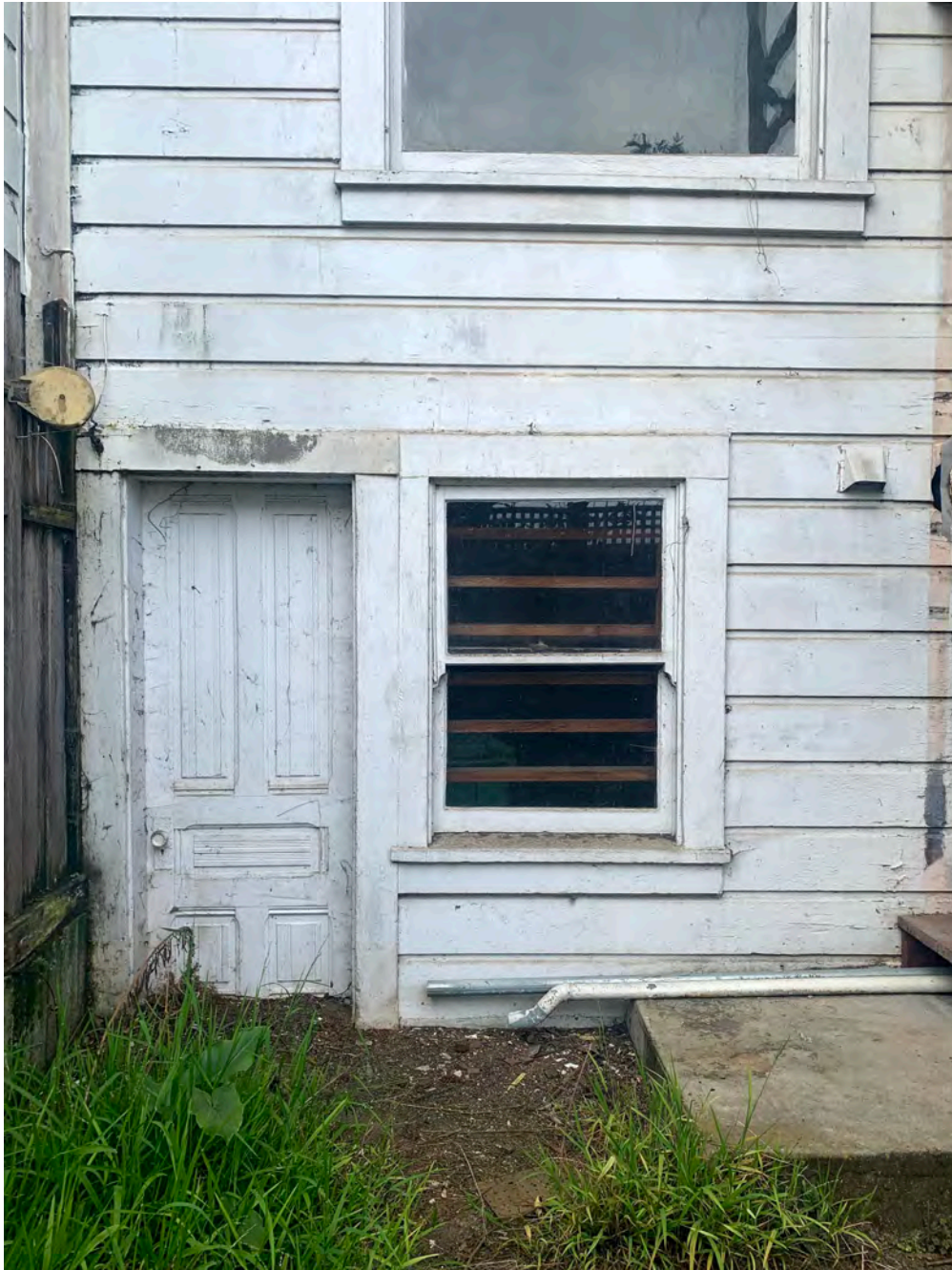
Photograph 27: Detail of rear, east façade, lower level with door, window and stair
