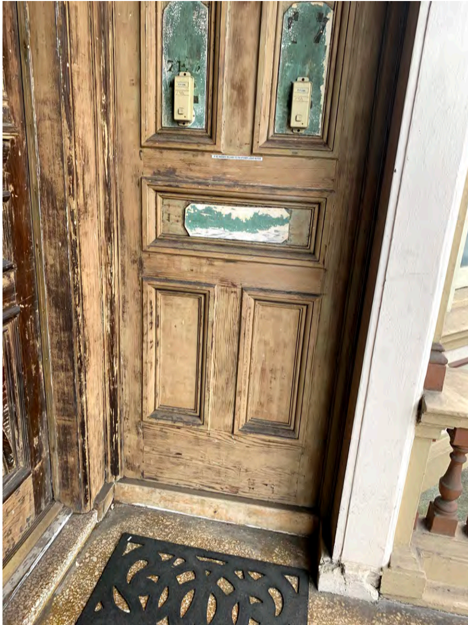
Photograph 11: 714 Steiner, primary Steiner Street façade, detail of wood paneling adjacent to front door.
