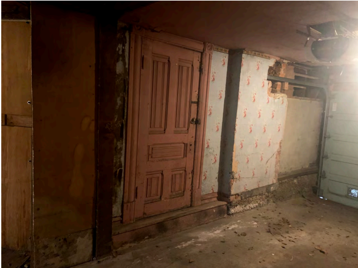
Photograph 54: South wall showing chimney condition with garage track damage.
