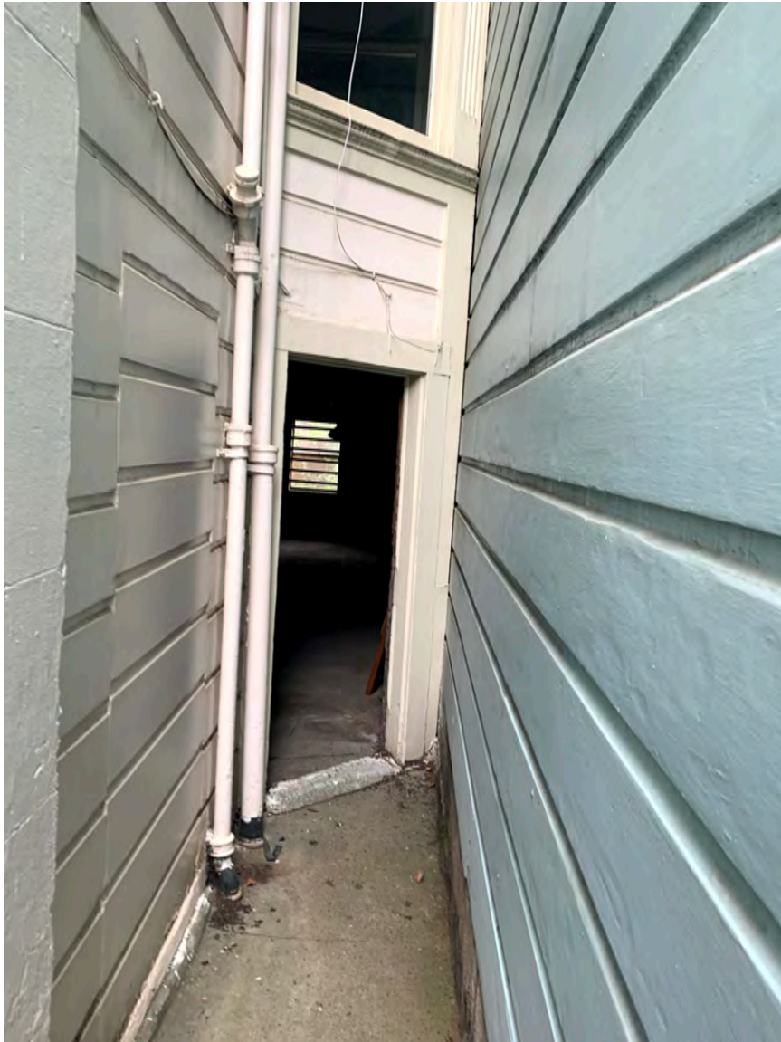
Photograph 23: 714 Steiner, south façade, detail of passageway between 714 and 712 Steiner with pedestrian door into garage and location of infilled door at left with mismatched patched siding and edge of chimney with scoring.
