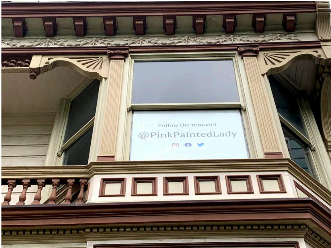
Photograph 20: 714 Steiner, primary Steiner Street façade, detail of upper story bay window and decorative detail
