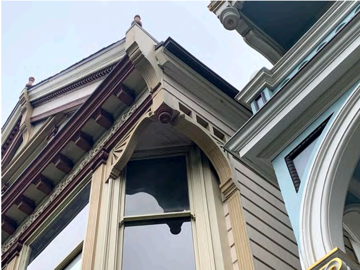
Photograph 21: 714 Steiner, primary Steiner Street façade, detail of angled bay window at upper story
