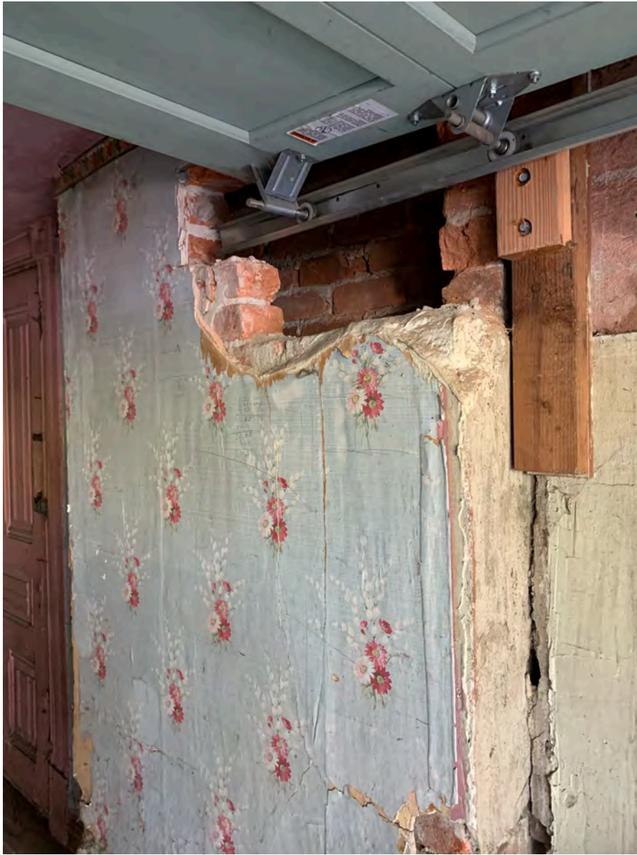
Photograph 53: South wall showing chimney condition with garage track damage.
