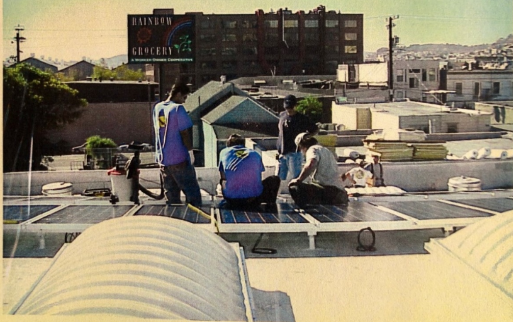
In 2002, Rainbow installed on our roof, what was then, the largest bank of photo voltaic solar panels in San Francisco.
