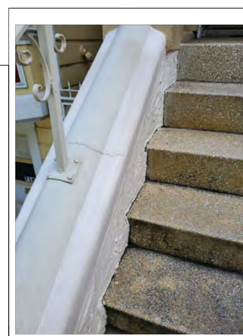
Photo 1: Existing brick framing where installation of garage door exposes damage to brick work. Large crack indicates separation between building and brick framing.
