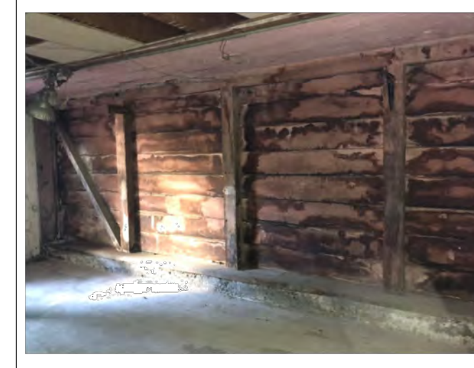
Photo 5: Existing first floor wall framing with water damage along south wall.
