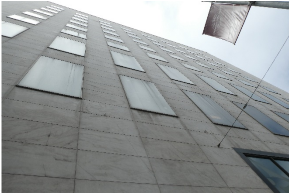
Figure 1: Photo of marble cladding. Note cracks in marble
