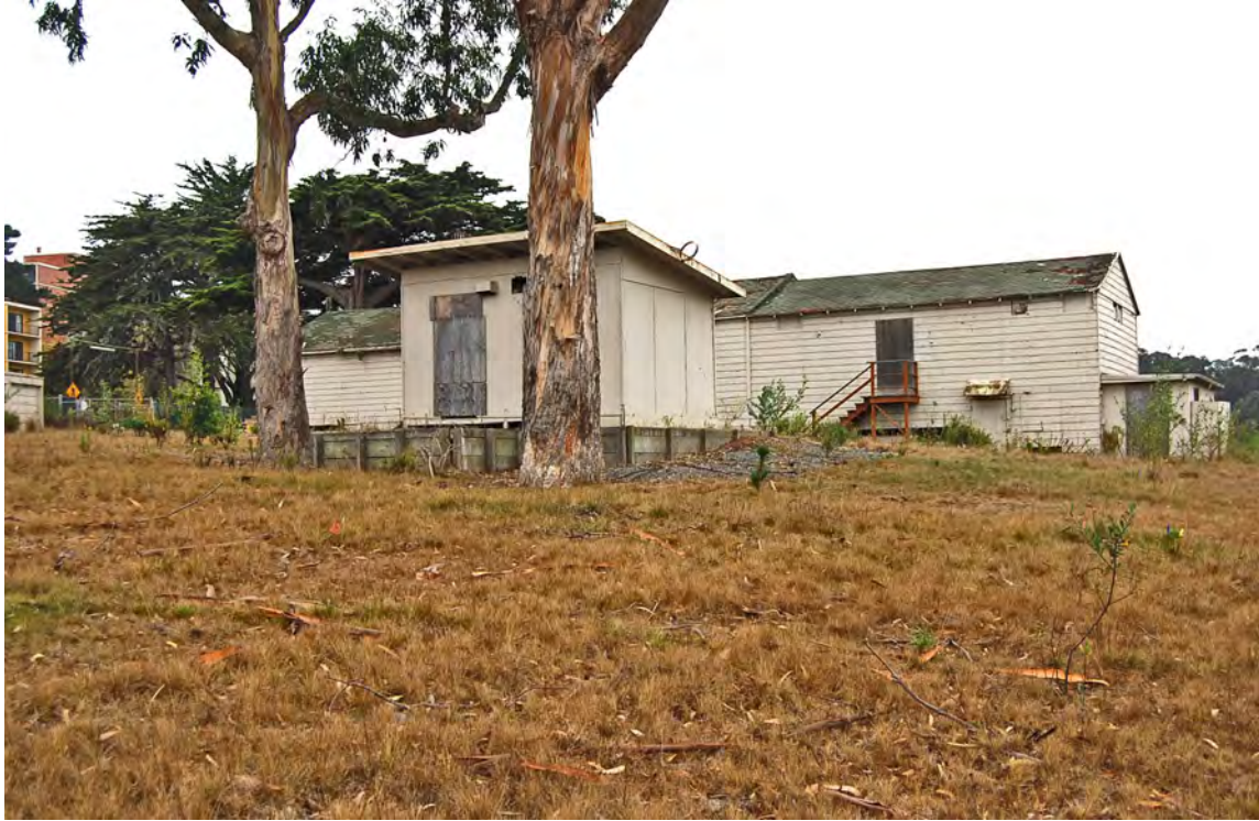
Photo 29. Barbeque Shed (non-contributing feature) with Rifle Range Building (contributing building) in background; facing west; 15 October 2019.
