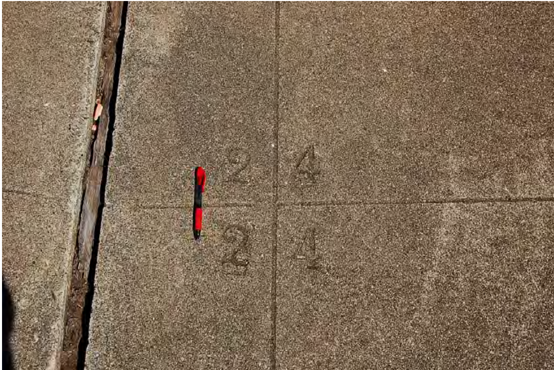
Photo 16. Detail of stamped distances for trap yardage markers found on the interior paved areas in Fields 4 to 7 (D. Bradley, September 2013).
