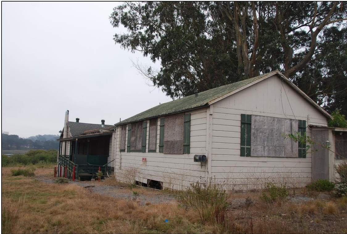
Figure 6: Caretaker's House (view southeast of west and north elevations). Note the Clubhouse is also visible in this photo.
