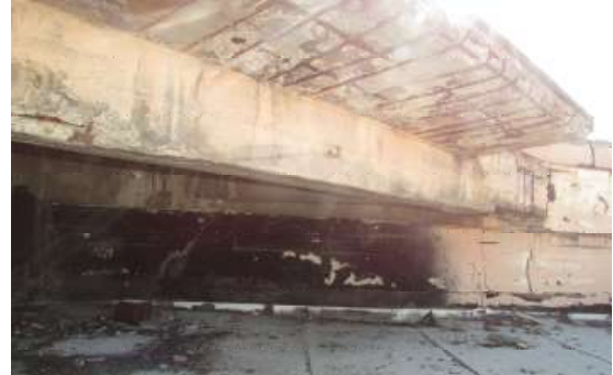
Figure 66. Extensive spalling and exposed reinforcement bar under the cantilevered extension of the tank-mount. Knapp Architects photo, 2019.
