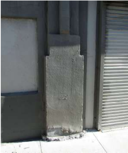
Figure 21. Tile column base that has been replaced by stucco in the same shape. Knapp Architects photo, 2019.
