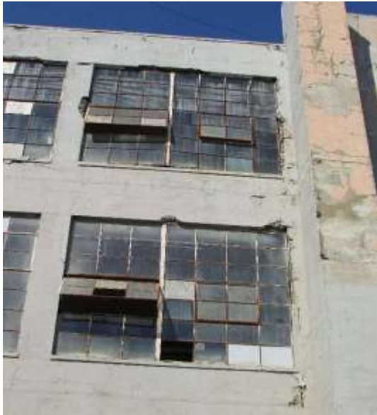
Figure 49. Spalls and cracks at the second and third floor windows in the third bay from the west. The incinerator smokestack is also visible at the right. Knapp Architects photo, 2019.
