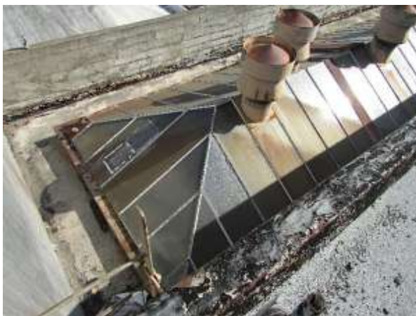
Figure 67. The large hipped skylight viewed from the main roof. It has extensive rusting of the metal frame and 40-50% broken or missing window putty. Knapp Architects photo, 2019.
