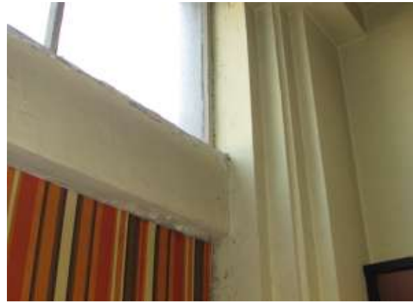
Figure 74. Visible leak damage and spalling at concrete window sill of 1 st floor front transom. Knapp Architects photo, 2019.
