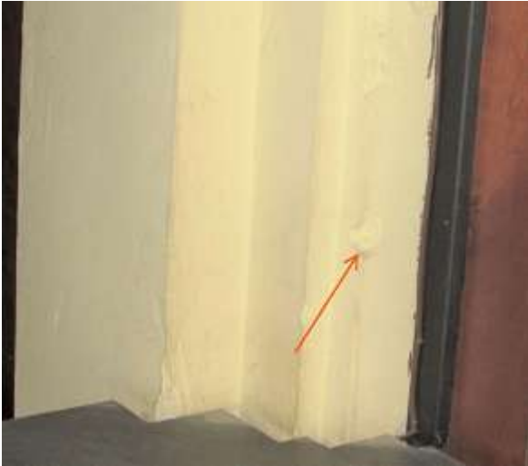
Figure 71. Interior stepped column with visible impact dents (red arrow). Knapp Architects
