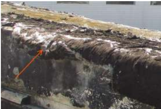
Figure 61. Hole in roofing over parapet showing exposed roofing (red arrow) Lichen is also visible. Knapp Architects photo, 2019.
