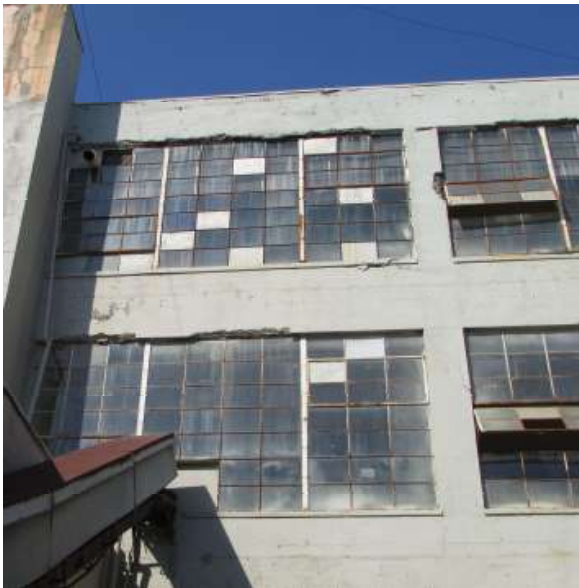
Figure 47. The distribution of cracks and spalls on the southern façade, at the second bay from the west. Knapp Architects photo, 2019.
