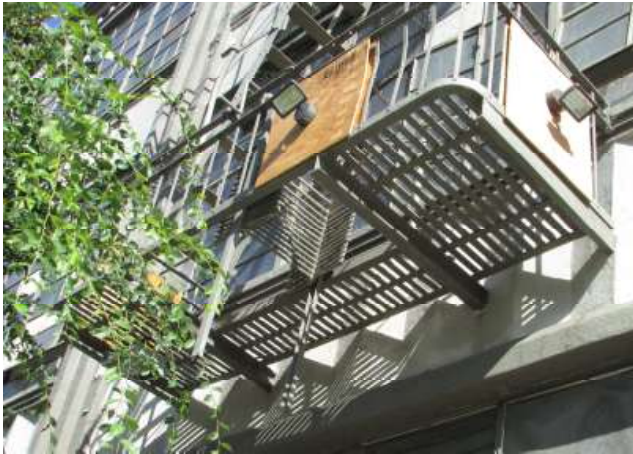
Figure 37. The Fire Escape attachments and the bottom of the fire escape at the third bay. Knapp Architects photo, 2019.
