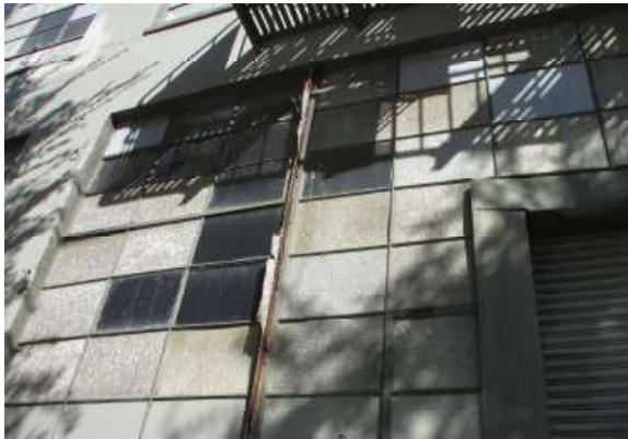
Figure 39. The central mullion of the first floor window in the second bay from the south, in the utilitarian section of the western facade, has rusted completely. Knapp Architects photo, 2019.
