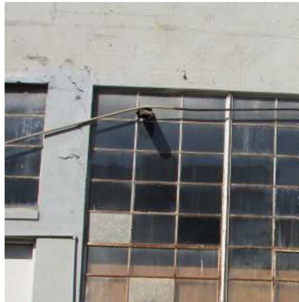
Figure 48. Extensive cracks at the upper west corner of the first floor window in the third bay from the west. Knapp Architects photo, 2019.
