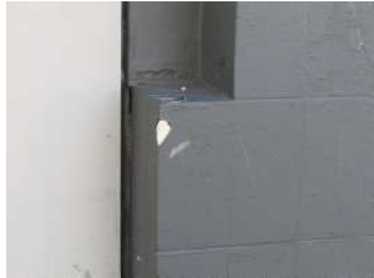
Figure 16. Chip on the tile column base at the north facade. Knapp Architects photo, 2019.
