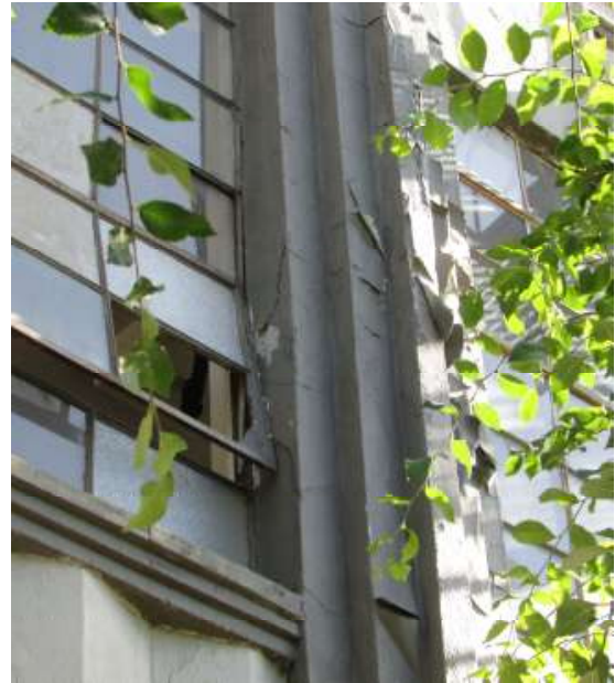
Figure 22. Crack from window traveling to the adjacent stepped column. Knapp Architects photo, 2019.
