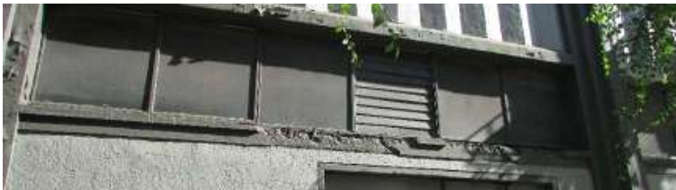
Figure 24. The transoms at the second bay from the north end of the west façade has a large spall at its sill. Knapp Architects photo, 2019.
