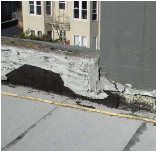
Figure 59. Typical view of roofing wrapping over the parapet. Holes and lichen are also visible on the top of the parapet. Knapp Architects photo, 2019.
