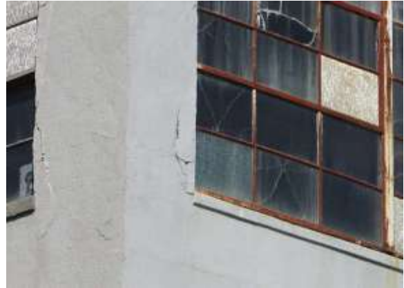
Figure 44. The third floor window of the westernmost bay has extensive cracking at its lower west jamb. Knapp Architects photo, 2019.
