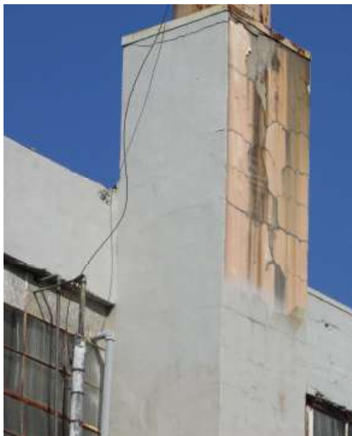
Figure 45. Cracks on the south facade of the Boiler Room smokestack. Knapp Architects photo, 2019.
