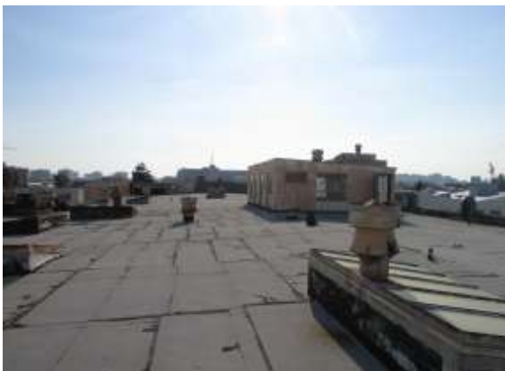
Figure 57. Roofing sheets with bitumen leaks at the northern part of the roof. Knapp Architects photo. 2019.
