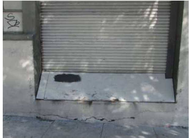
Figure 38. There is an extensive crack in the wall below the loading dock at the south end of the west façade. Knapp Architects photo, 2019.
