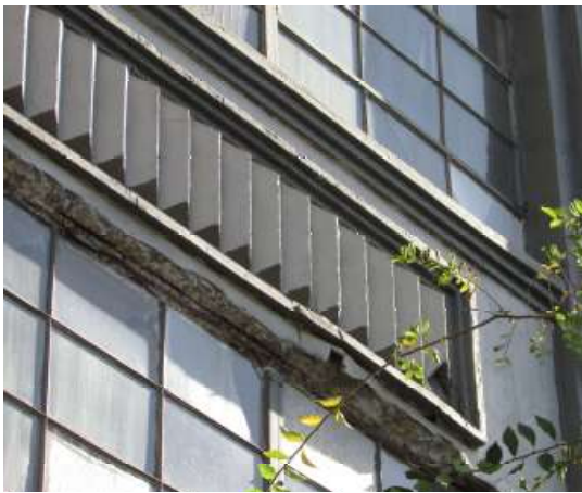
Figure 29. The spall at the window has spread to cracks in the spandrel. One spandrel angle is broken at the bottom. Knapp Architects photo, 2019.
