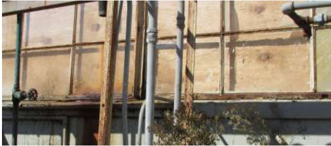
Figure 55. The first floor window, in the fourth window bay from the west has extensive rust, especially at the sill. Knapp Architects photo, 2019.
