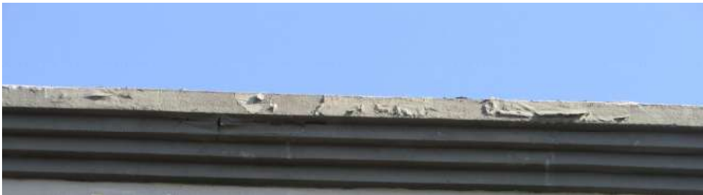
Figure 33. Typical condition of the stepped cornice at the Russ Street façade. Knapp Architects photo, 2019.
