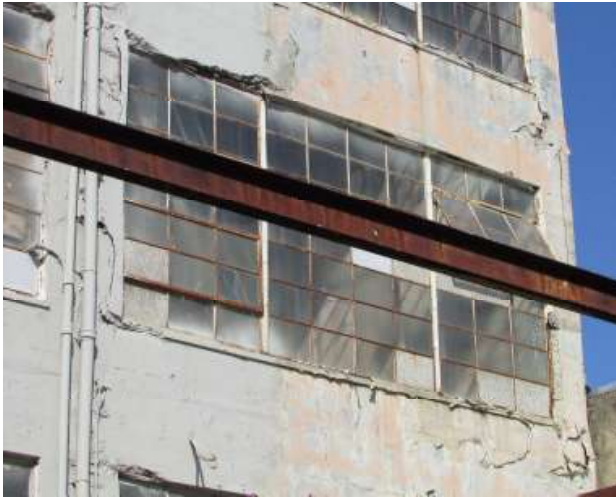
Figure 53. Spalls and cracks at the second floor window of the easternmost window bay. Knapp Architects photo, 2019.
