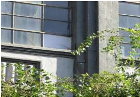
Figure 26. The northernmost bay of third floor windows on the west façade has a crack at the bottom of the south jamb. Knapp Architects photo, 2019.
