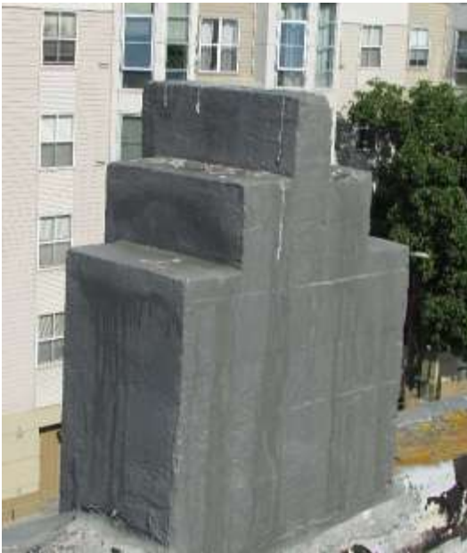
Figure 63. The backs of the stepped capitals are generally in good condition. Knapp Architects photo, 2019.
