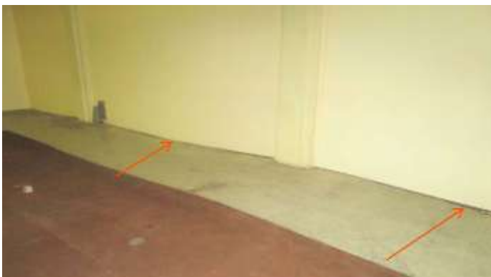
Figure 72. Visible settling of the floor between columns, in the front office section (red arrows). Settling is as much as four inches below the level next to the columns and the floor is coming away from the wall base at the right red arrow. Knapp Architects photo, 2018.
