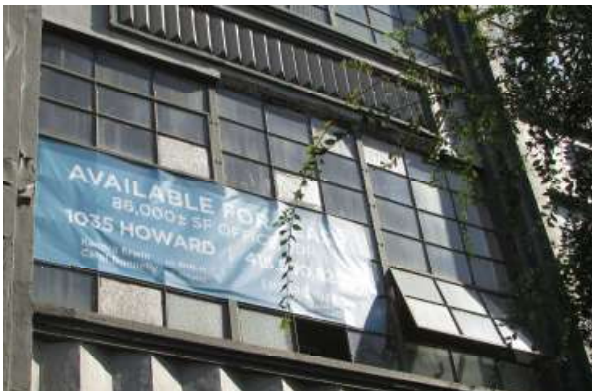
Figure 34. The first bay of second floor windows on the west façade has a 65% spall by length at the head, and there are 35% missing, painted or fiberglass windows. Knapp Architects photo, 2019.
