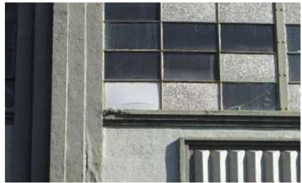
Figure 27. A one square foot spall at the north end of the sill in the third floor fifth bay window. Knapp Architects photo, 2019.
