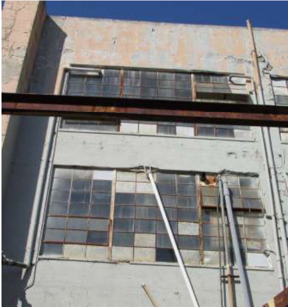
Figure 51. The second and third floor windows in the fourth window bay from the west. Knapp Architects photo, 2019.
