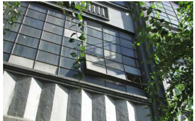
Figure 35. The operable portion of the second floor window at the second bay appears twisted in its frame and not properly closeable. Knapp Architects photo, 2019.
