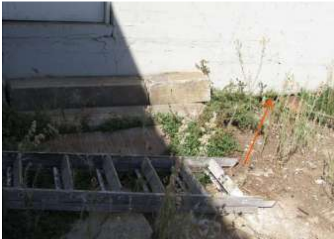
Figure 41. A substantial gap occurs between the bottom of the southern façade and the adjacent grade (red arrow). Knapp Architects photo, 2019.
