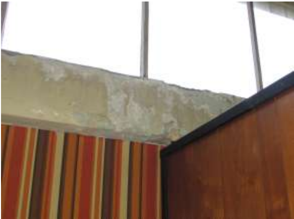
Figure 73. Visible leak damage and spalling at concrete window sill of 1 st floor front transom. Sealant has been applied to the exterior frames to stop the leakage, but the concrete damage remains. Knapp Architects photo, 2019.
