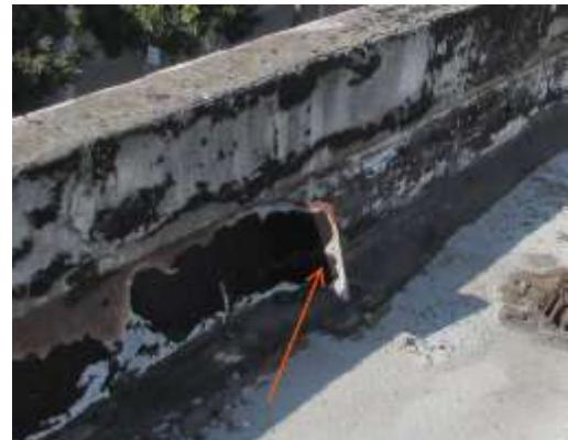
Figure 62. Rusty roof flashing that has become detached and bent away. Knapp Architects photo, 2019.
