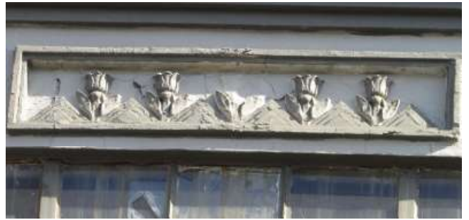
Figure 32. The Tulip at the center and the frame are spalled. Knapp Architects photo, 2019.
