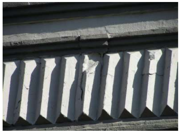
Figure 30. Spalls and cracks in the second bay from the north end of the Russ Street facade. Knapp Architects photo, 2019.
