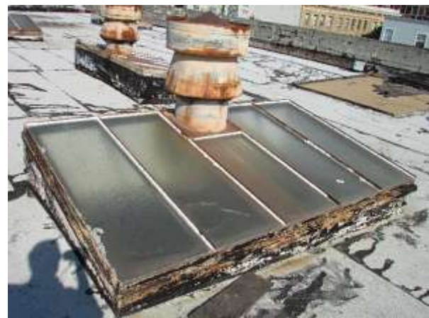
Figure 68. A typical small skylight. It exhibits light rusting at the frame, light rusting on the roof vent and 40% broken putty. Knapp Architects photo, 2019.
