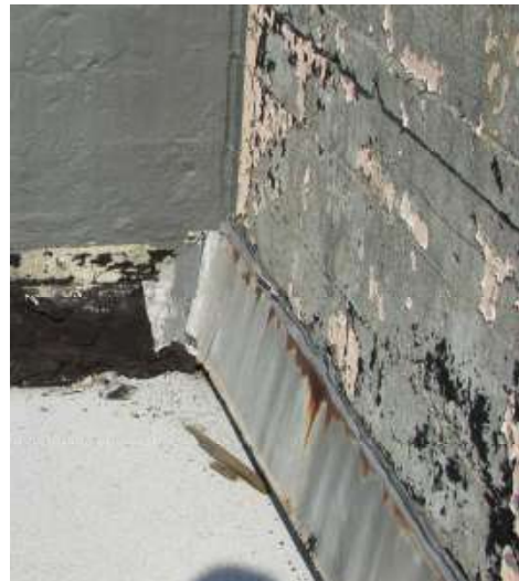
Figure 60. Typical view of roofing terminated by counter-flashing at the bottom of the parapet. Knapp Architects photo, 2019.
