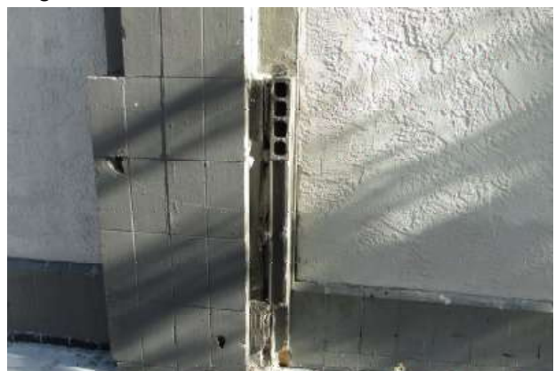
Figure 20. Column base with the tiles missing at the corner. Knapp Architects photo, 2019.
