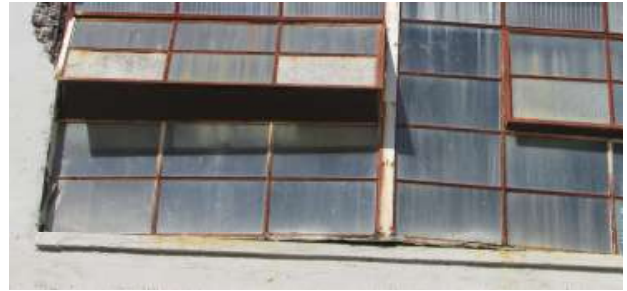
Figure 56. The base of the central mullion is detached about two inches from the frame sill of the third floor window in the third window bay from the west. Knapp Architects photo, 2019.
