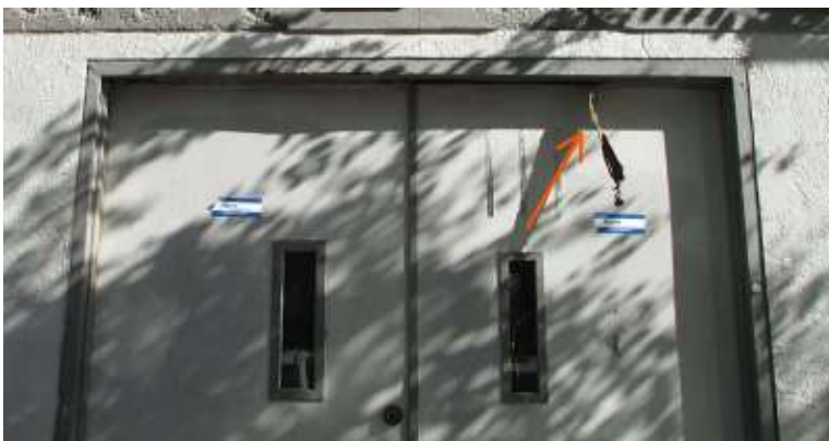
Figure 36. The head of the door at the north end of the western façade has a frame that is extensively rusted and is peeling away (red arrow). The adjacent wall is in good condition. Knapp Architects photo, 2019.
