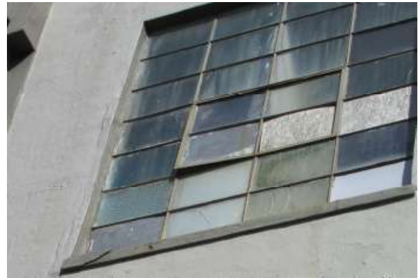
Figure 40. The operable portion of the northernmost window of the utilitarian section of the Russ Street facade at the third floor appears twisted in its frame and unable to close. This view also shows a typical distribution of opaque, painted or fiberglass panes. Knapp Architects photo, 2019.
