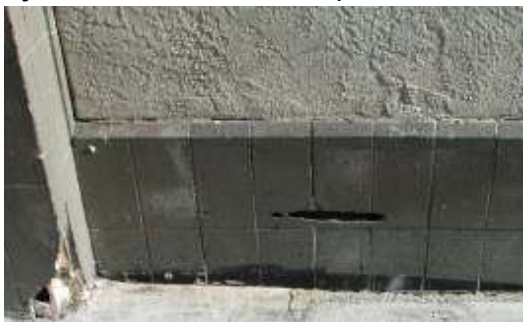
Figure 19. Holes in the base tile at the Russ Street façade. Part of the original black terra cotta glazed surface is visible at the tile bottoms. Knapp Architects photo, 2019.
