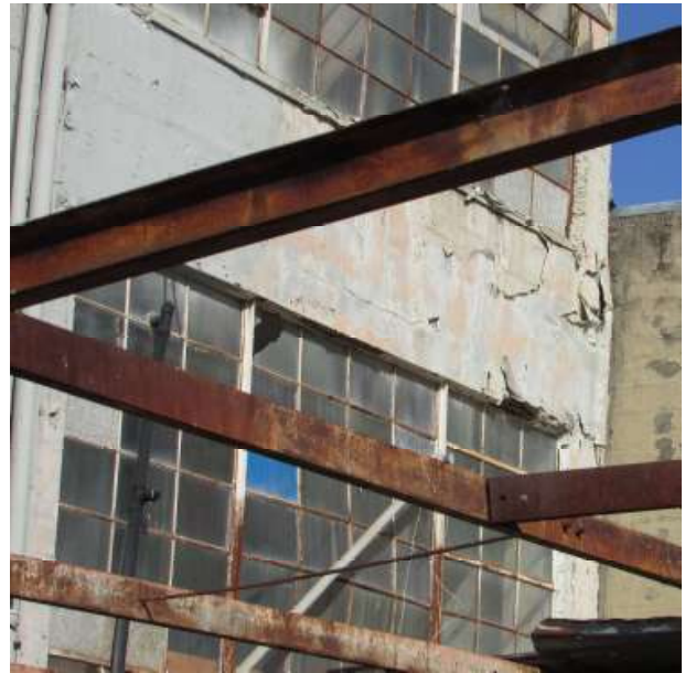
Figure 52. The first and second floor windows in the easternmost bay. Knapp Architects photo, 2019.
