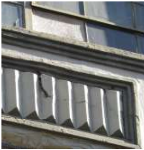
Figure 31. A crack extends across four ribs between the second and third floors of the western facade. Knapp Architects photo, 2019.
