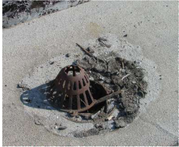
Figure 70. Partially detached roof drain. Knapp Architects photo, 2019.
