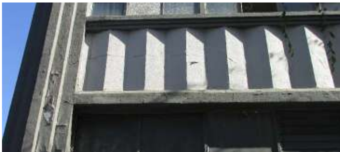
Figure 28. Crack across accordion ribs of a spandrel panel between the first and second floors, at the north end of the Russ Street facade. Knapp Architects photo, 2019.
