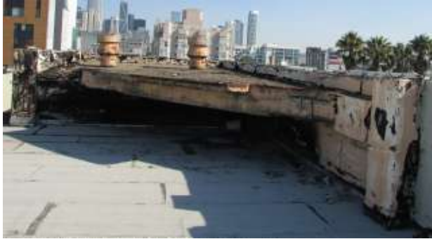
Figure 65. The five-sided, tank-mount structure at the southeast corner of the roof. Knapp Architects photo, 2019.
