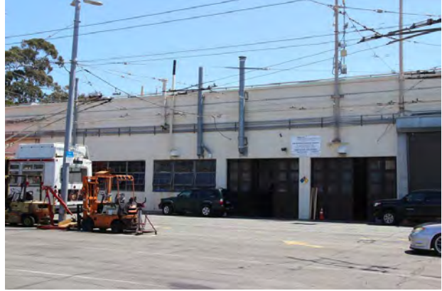
Figure 50. Older windows and doors on west façade, looking northeast from bus yard.
