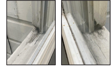
PHOTOS OF EXISTING WINDOW AT KITCHEN BAY SHOWING DETERIORATION AND CAN NO LONGER BE OPENED
