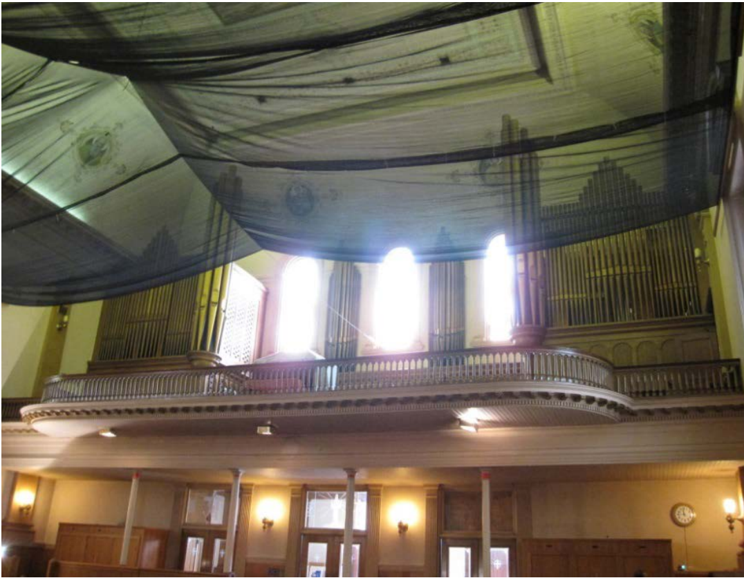
Photo 2. Choir loft with organ intact, view west, 2009. Note that the organ at the left side of the choir loft extends out from the west window wall and the opening to the connector is not visible (photo courtesy of Chris VerPlanck).
