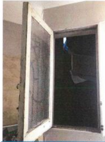
Air and light to bathroom blocked
