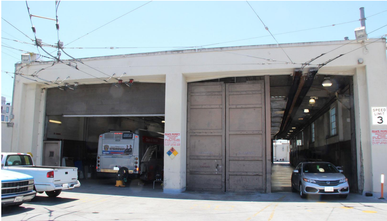
Figure 45. North façade of second floor maintenance shops, looking south from parking deck.
