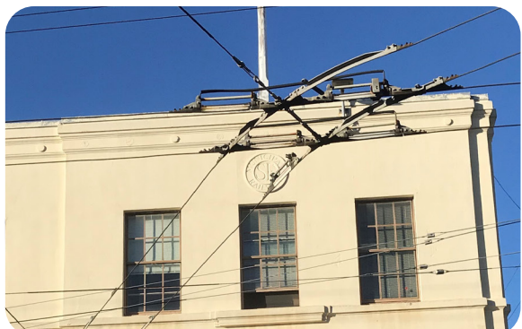
Image 6: Detail view of office wing primary façade. Note character defining features including molded concrete and cement plaster ornament, fenestration pattern of groups of three double-hung metal windows, medallion featuring original Muni logo, and flagpole
