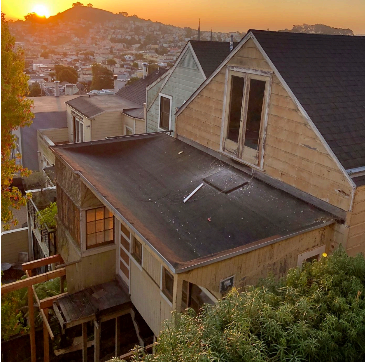
This photo is from October 2019. It shows the roof (without a deck) prior to the new construction.
