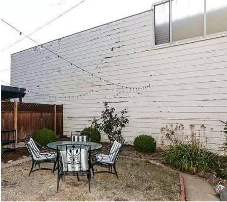
Existing Photo from Rear Yard of 41-43 Mallorca Way with Existing 25 Toledo Way 20' Wall
