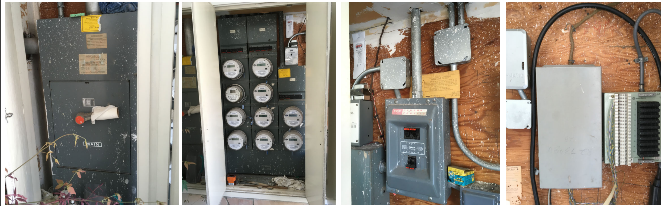
600A MAIN DISCONNECT SWITCH (QMQB UNIT - 7032)
