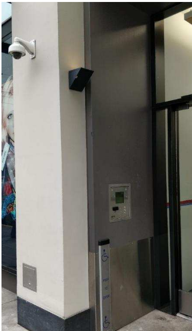
Figure 6 (Entry with Handicap Accessible Door Actuator & Card Reader on Building Intercom)
