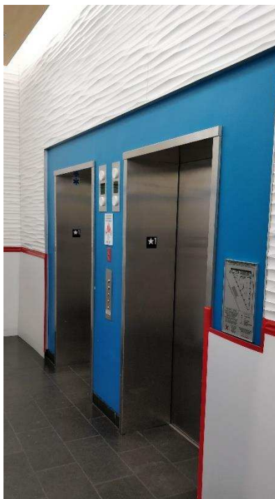
Figure 11 (Two (2) Elevator Cabs)
