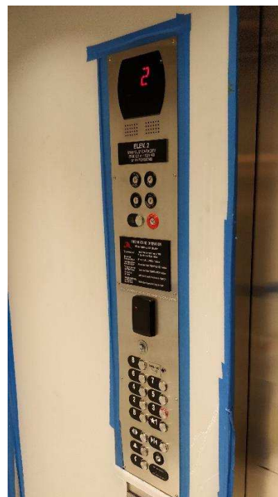
Figure 12 (Card Reader Inside Elevator)
