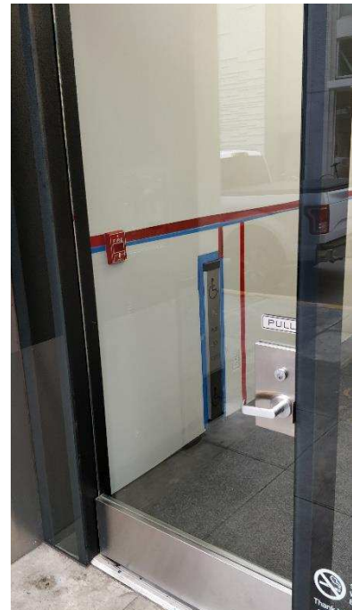
Figure 7 (Inside Lobby Handicap Accessible Door Actuator)
