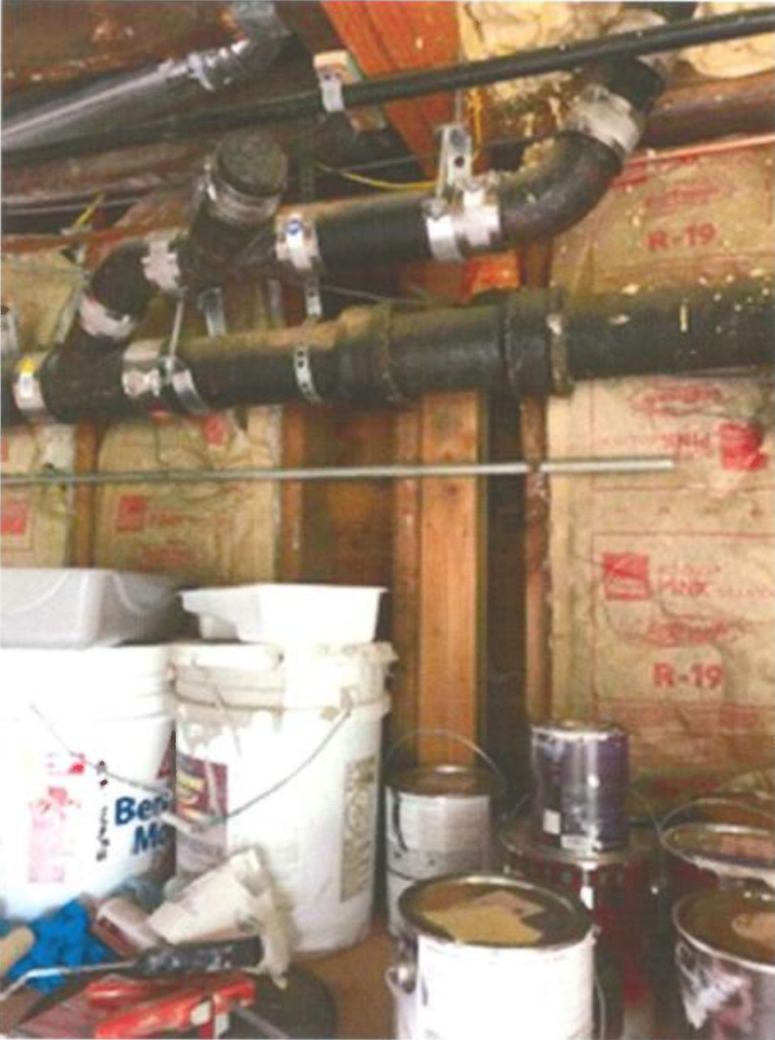
Shared Wall and Sewer Line Viewed from the Basement Level of the Platzman Rear Building
