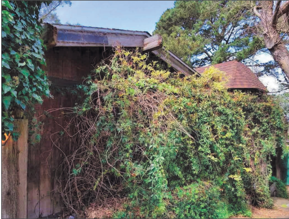
1043-1045 Clayton Street – View west of the northern portion of the east elevation (primary façade), (image courtesy of HRE Part 1 prepared by Tim Kelley, p. 6)
