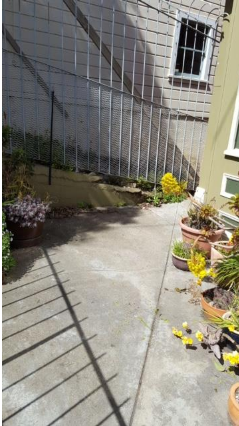
Damaged wall near front of our home
