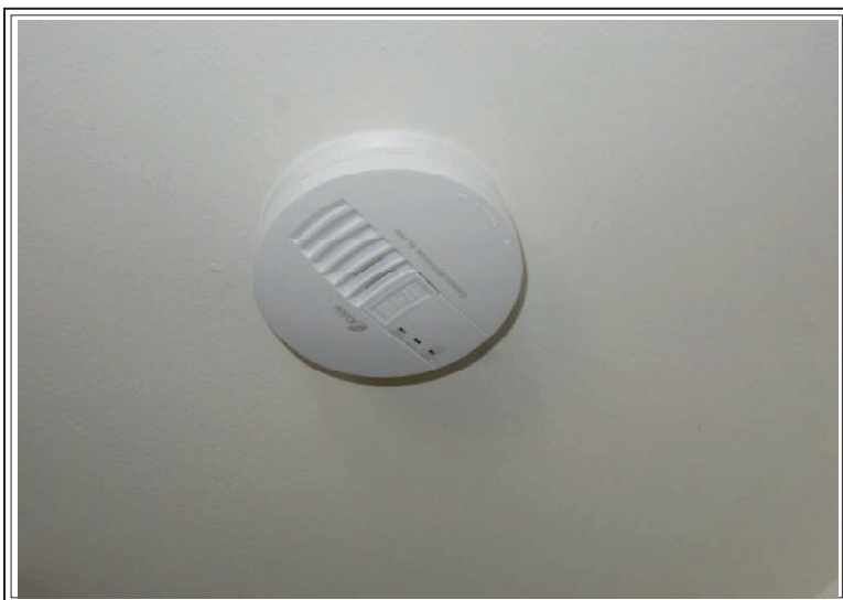
Unit#376-A Smoke And Carbon Monoxide Detector
