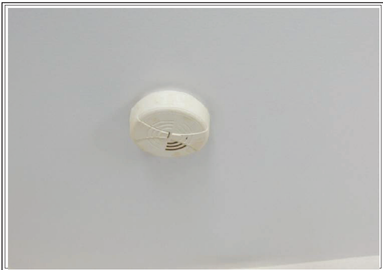
Smoke And Carbon Monoxide Detector
