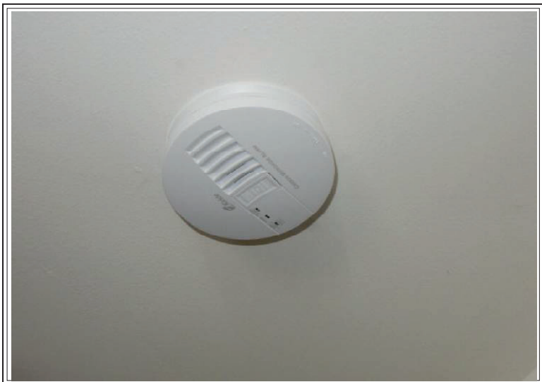
Smoke And Carbon Monoxide Detector
