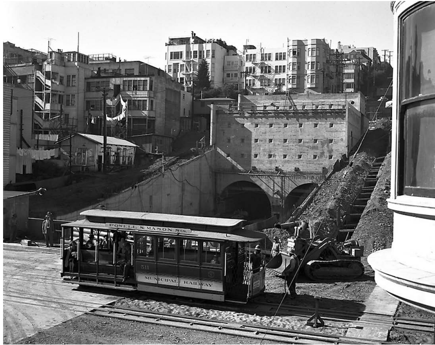
Construction of the Broadway Tunnel at Powell Street, November 5, 1951 SFMTA Photographic Archive
