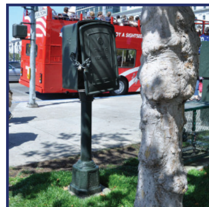
Traffic control box at Fulton and Larkin Streets
