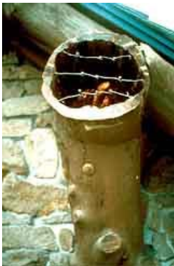
The core of a deteriorated wood outrigger was first drilled out. Photos (left and right): Courtesy, Harrison Goodall.
