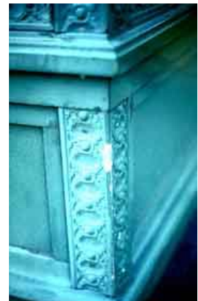
Substitute materials need to be located with care to avoid damage. The fiberglass column base has chipped, whereas the historic cast iron would have remained sound. Photo: NPS files.
