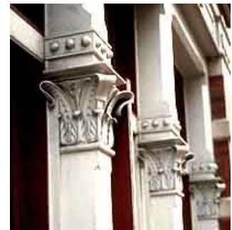
Cast aluminum used as a replacement for cast iron. Photo: NPS files.
