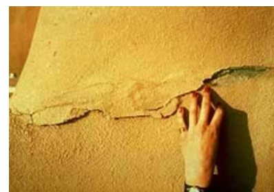
A waterproof coating is an inappropriate substitute material to apply to adobe as it seals in moisture and may result in spalling. Photo: NPS files.
