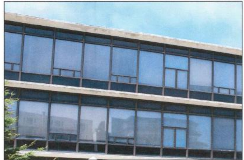
Glass curtain wall composed of bronze powder coated aluminum framing system in a regularly spaced pattern of mullions and muntins, typically with a small spandrel panel of obscure glass below a larger pane.
