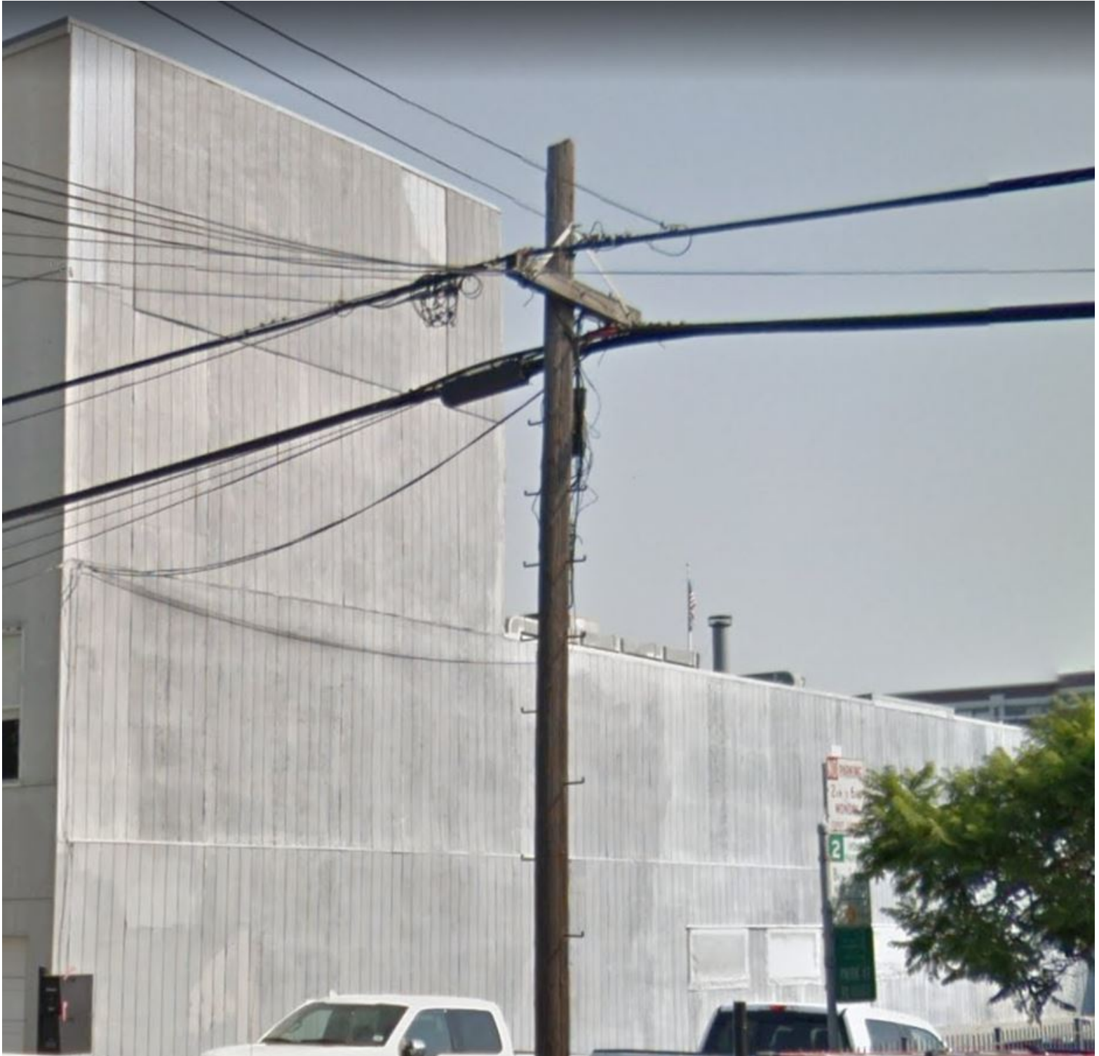
South elevation displaying the existing cladding proposed for removal and replacement.
