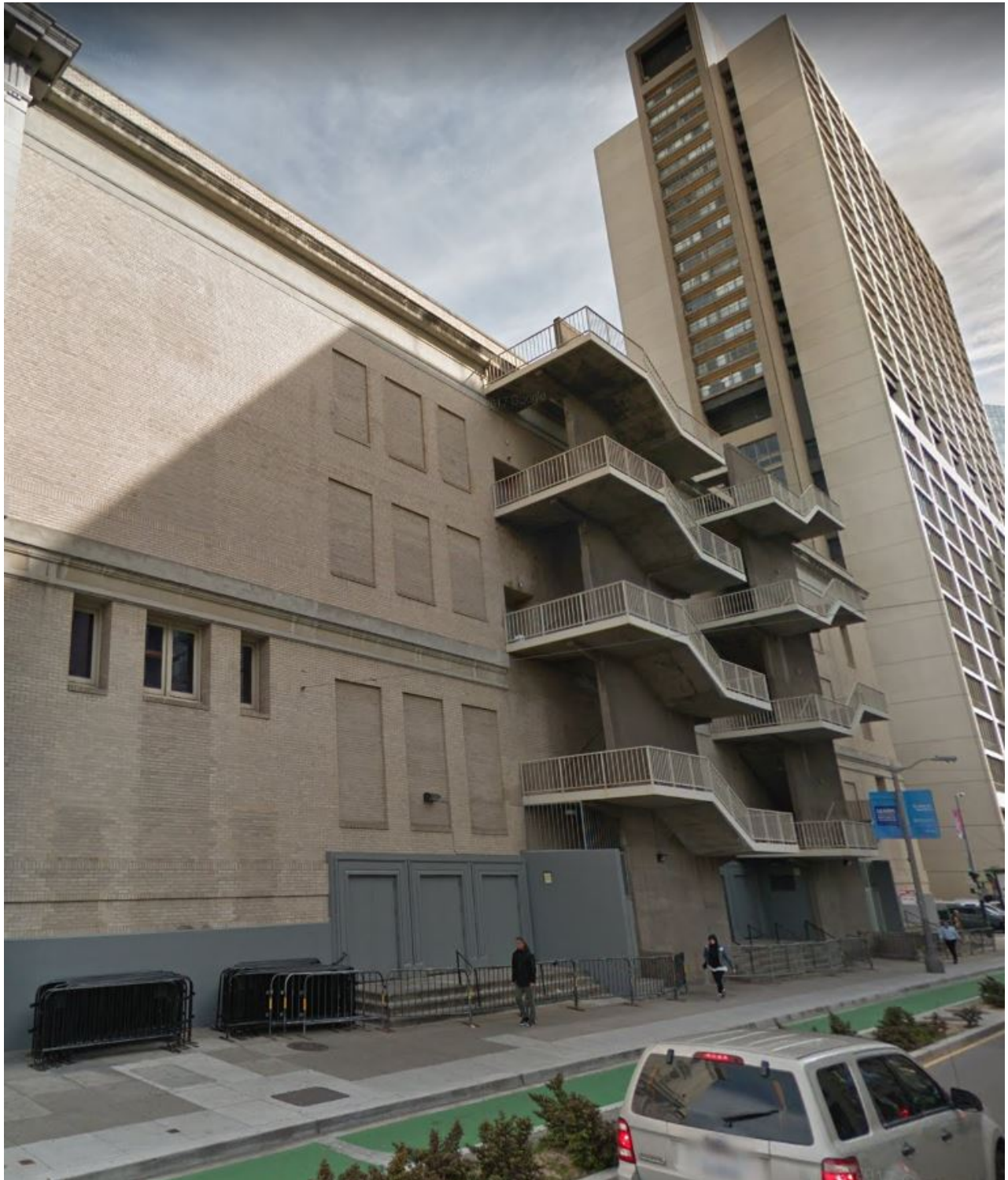
*Area of work is limited to the depicted brick portion of the western façade.
