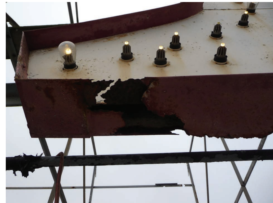
Photo of corrosion at bottom of the letter, at the front and back, and missing glass bulbs
