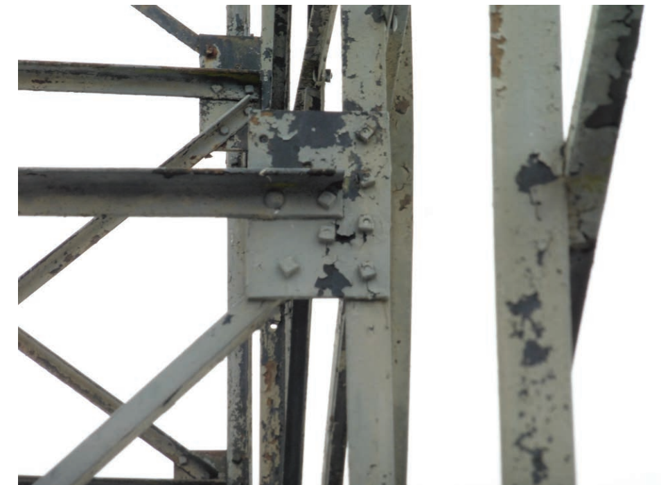
Photo of typical connections and members in the steel truss frame, showing corrosion and loss of paint
