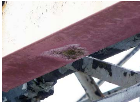
Figure 7 - Moderate deterioration at this weep hole in the form of corrosion with associated paint deterioration.
