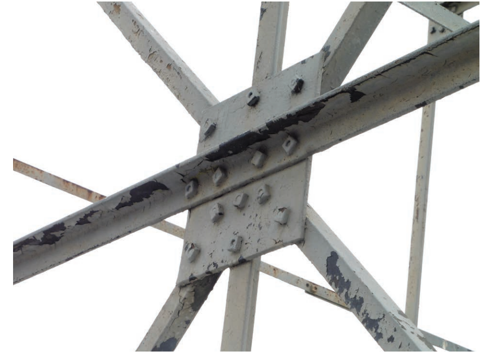
Photo of typical connection in the steel truss frame, showing corrosion and loss of paint
