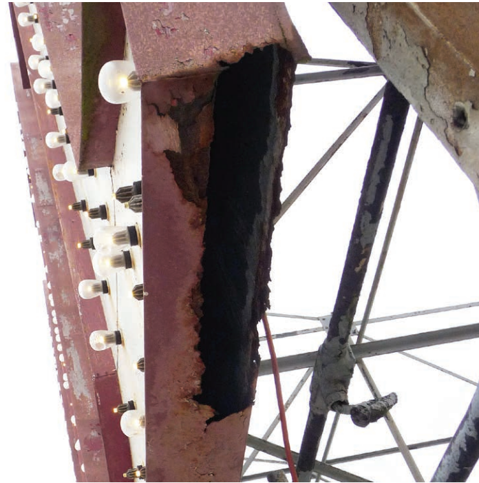
Close up of back side of letter showing corrosion at the bottom of the letter
