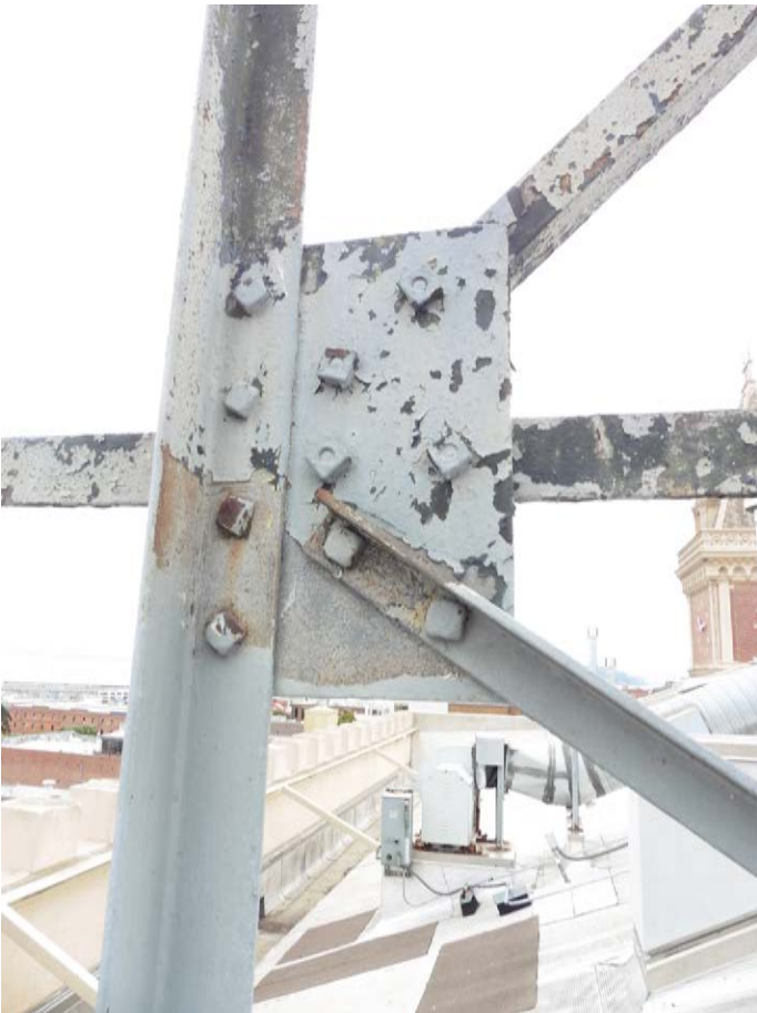
Figure 16 - A typical "fair" condition connection of the armature, on the lower roof (Mustard Building), above arm's reach
