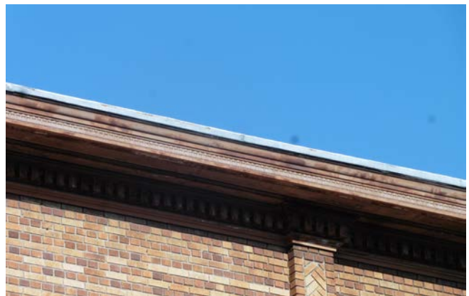
Figure 4. Corrosion along cornice edge on west.
