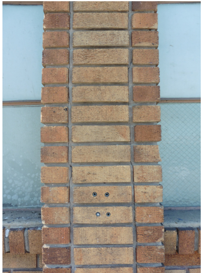
Figure 5. Typical condition of brick at south & west walls, clean all surfaces prior to further rehabilitation work.
