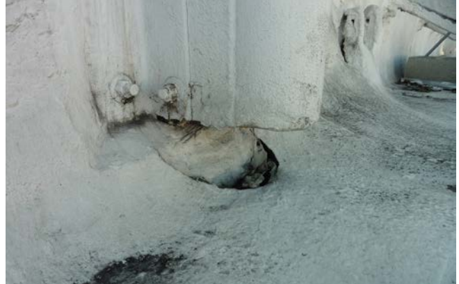
Figure 3. Detail of flagpole anchor; note corrosion and damage to roofing, even after re-roofing.
