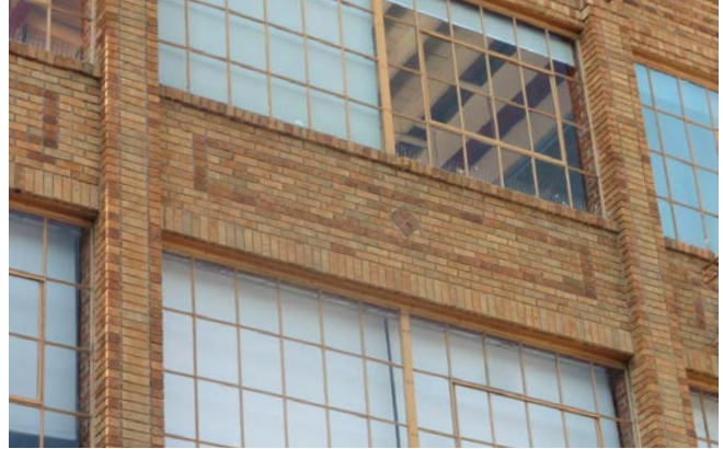
Figure 3. South elevation; note recessed mortar joints to be maintained and replicated in re-pointing.
