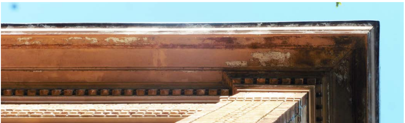
Figure 3. Cornice at southwest corner; localized areas of severe damage observed & requiring immediate repair.
