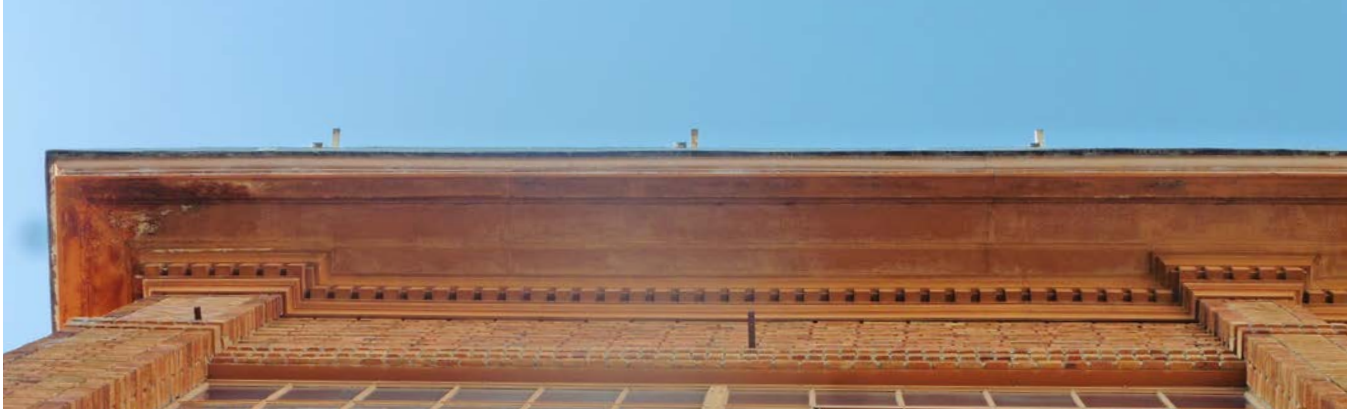
Figure 2. Cornice along west; note discoloration and localized corrosion, conditions are considered typical.
