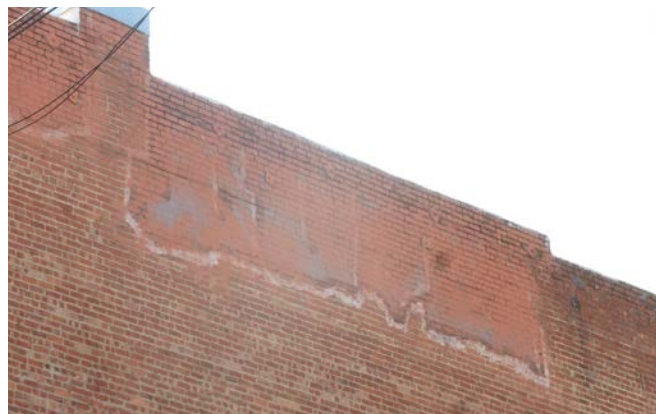
Figure 2. East Elevation; note graffiti & paint to be removed.
