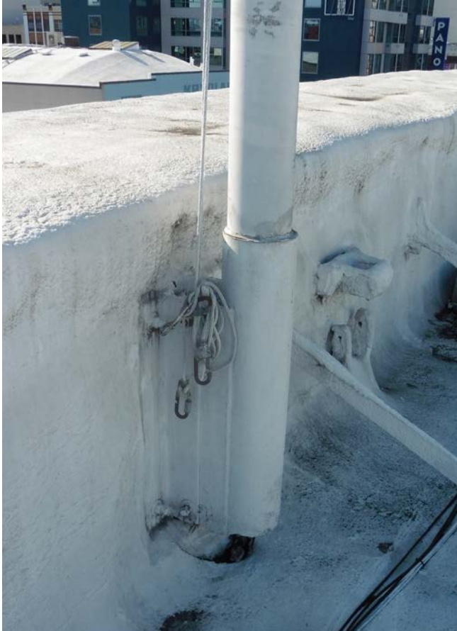
Figure 2. Flagpole anchor; note fastener conditions and localized signs of corrosion.
