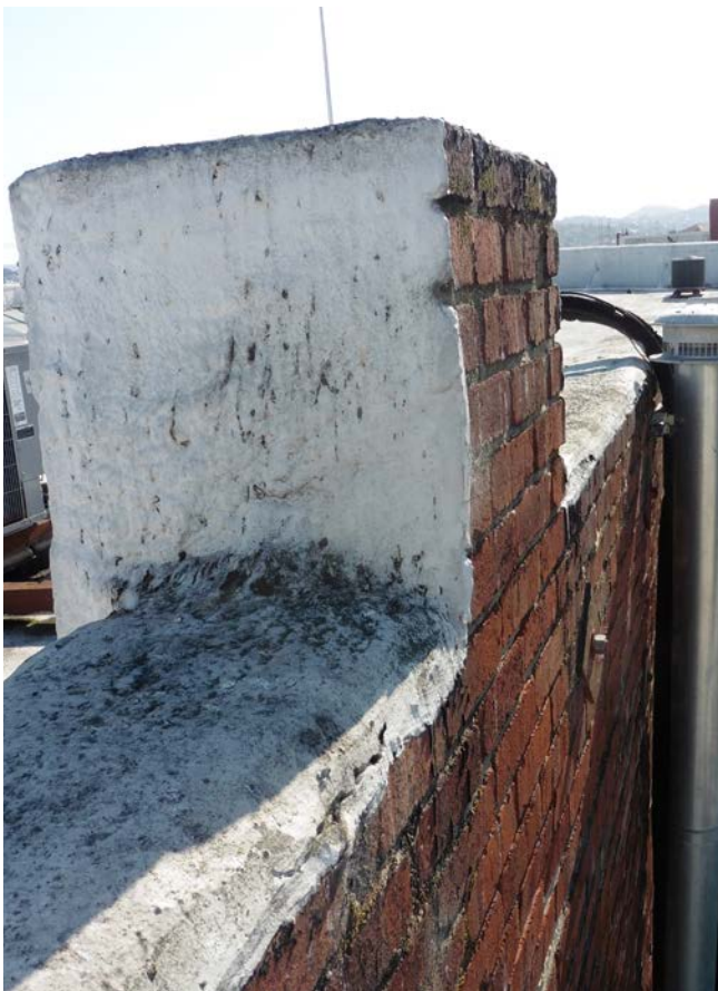
Figure 3. Unbraced ventilation stack at north wall.
