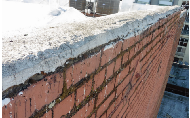
Figure 5. East elevation at roof parapet; note bio-growth and discoloration to be addressed prior to rehabilitation work.
