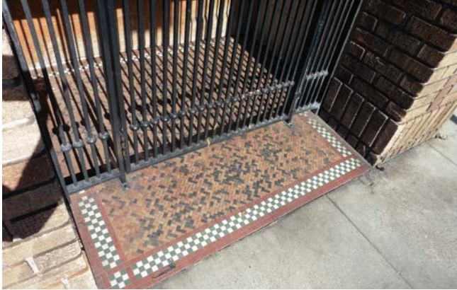
Figure 2. Entry tiling. Entry gate has been added.
