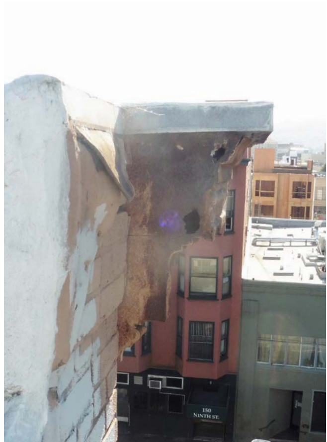
Figure 1. Cornice at northwest corner; note level of corrosion, this is worst condition observed and atypical of overall cornice.
