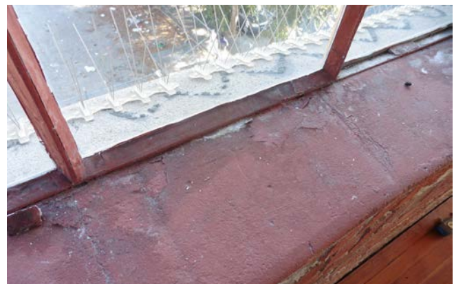
Figure 2: Concrete parge at south window sills, typical. Note level of localized cracking and paint deterioration.
