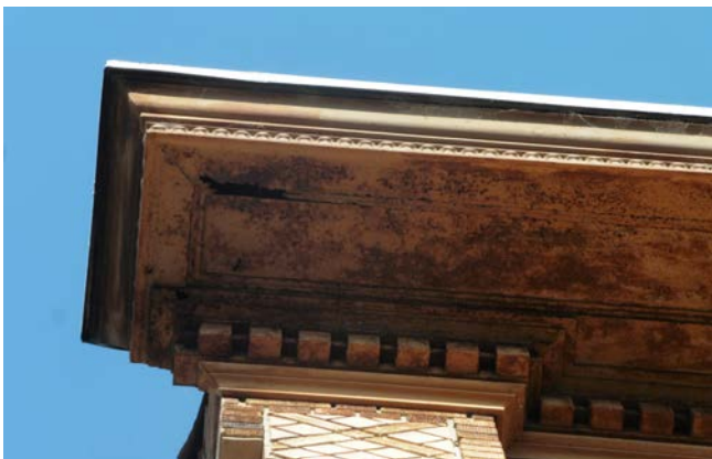
Figure 3. Cornice at northwest corner; localized areas of severe damage observed & requiring immediate repair.
