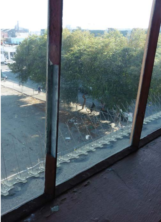
Figure 3. Steel window frame detail and glazing putty loss.
