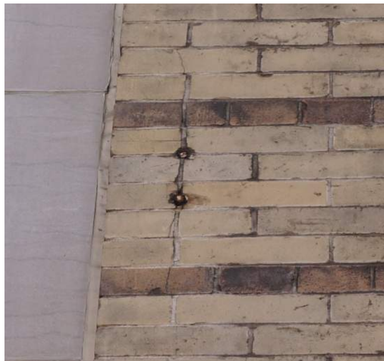
17-29 Third Street - Holes with old attachments, cracked brick and mortar joints.
