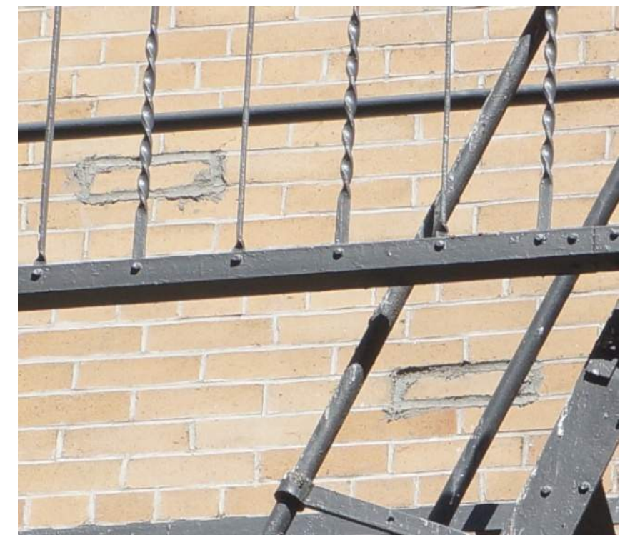
17-29 Third Street - Limited locations of mismatched mortar
