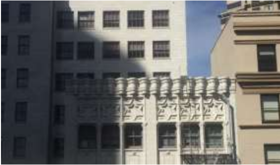
Top floor of the Annex (190 Stevenson Street), south elevation. (Knapp Architects photograph.)
