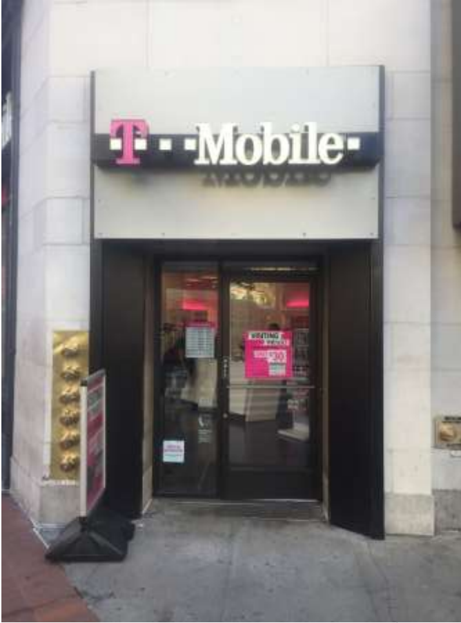
Entrance to T-Mobile store on Third Street, at corner of Market Street. Note non-original sheet metal surround and sign panel over door; original door surround and transom are believed to exist underneath. (Knapp Architects photograph.)
