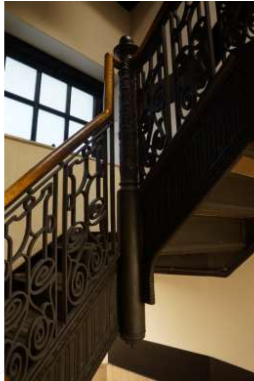
Main stair, typical upper run with cast iron pans. (Knapp Architects photograph.)
