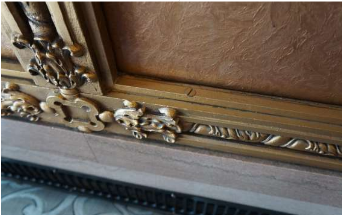
The embossed gold panels are mounted on glass, which is held in place by stops in the bronze grid in which the panels lie. Screws secure the stops. (Knapp Architects photograph.)
