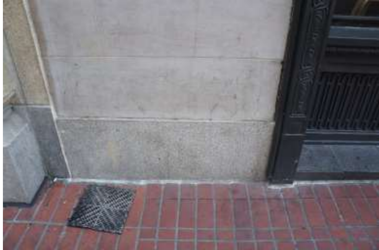
Granite base course and marble cladding above are visible at center; cast iron jamb of storefront surround and bulkhead are visible at right. (Knapp Architects photograph.)
