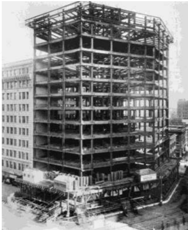
Construction of the Hearst Building, ca. 1909. Note framing for original sheet metal cornice. Courtesy the Hearst Corporation.
