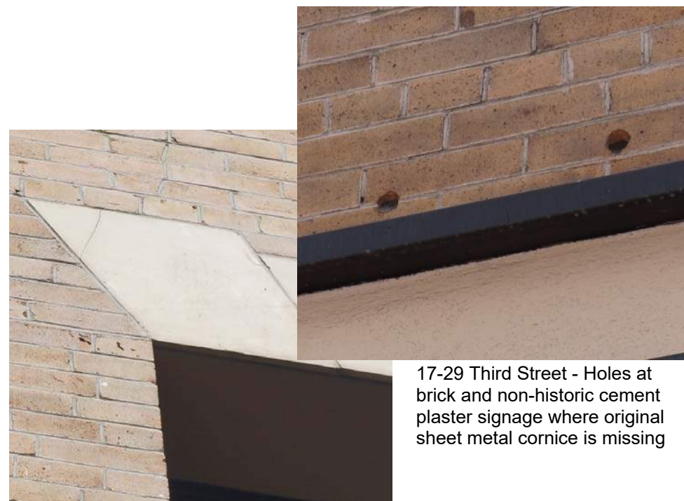
17-29 Third Street - Minor hairline crack at terra cotta
