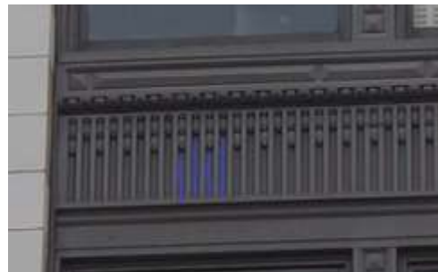
Typical spandrel panel in cast iron at upper floors. (Knapp Architects photograph.)
