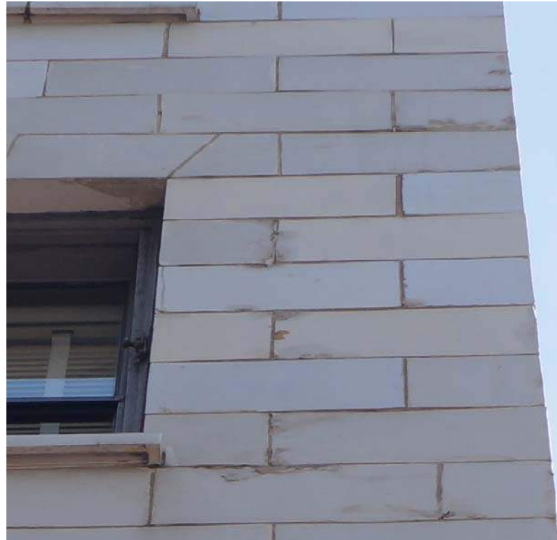
Hearst Building - Loose glazing and glaze spalls in limited
