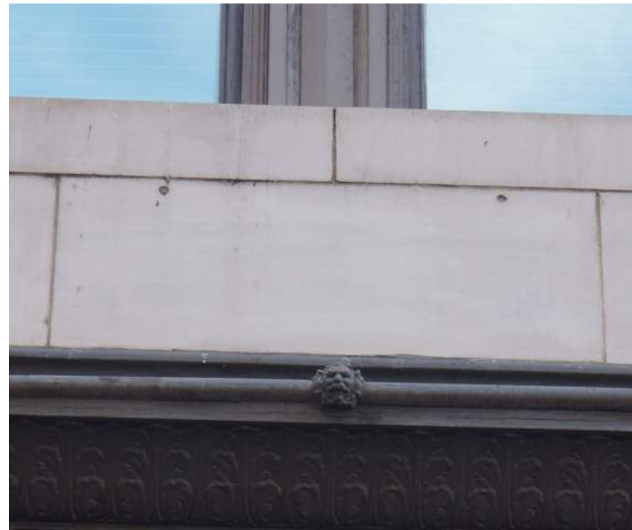
Hearst Building – Minor previously patched holes mismatched with surrounding terra cotta glaze
