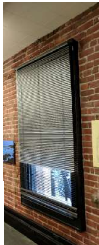
As viewed from the interior (right), the window frames at the upper floors of 17-29 Third Street protrude from the face of the brick wall. This and what appear to be remnants of plaster indicate the original interior finish was plaster, which has been removed. (Knapp Architects photograph.)
