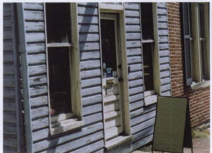
Figure 8. The paint on the siding of this south-facing wall needs to be scraped, sanded, primed and repainted. Postponing such work will lead to further paint failure, require greater preparatory costs, and could even result in the need to replace some siding. Photo: Charles Fisher.
