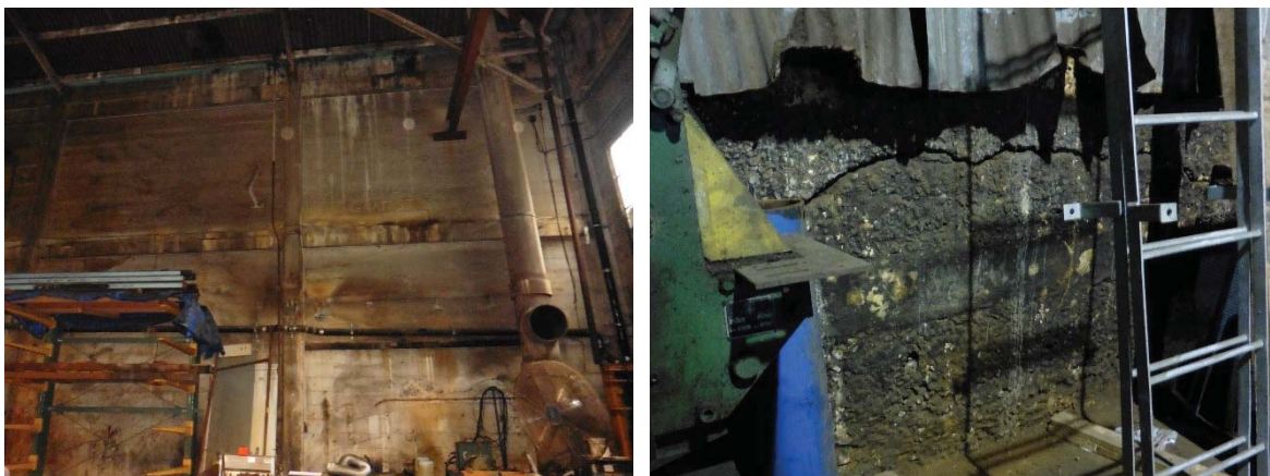
Figure 16: (Left) The rear (northwest) board-formed concrete wall of the east warehouse space with heavy corrosion staining; (Right) Large horizontal crack through the rear (northwest) low concrete wall of the west warehouse space.
