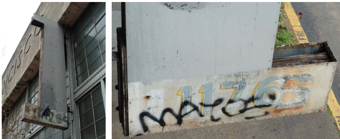
Figure 7: (Left) East side of blade sign; (Right) View of lower part of blade sign from above showing deterioration of wood core.
