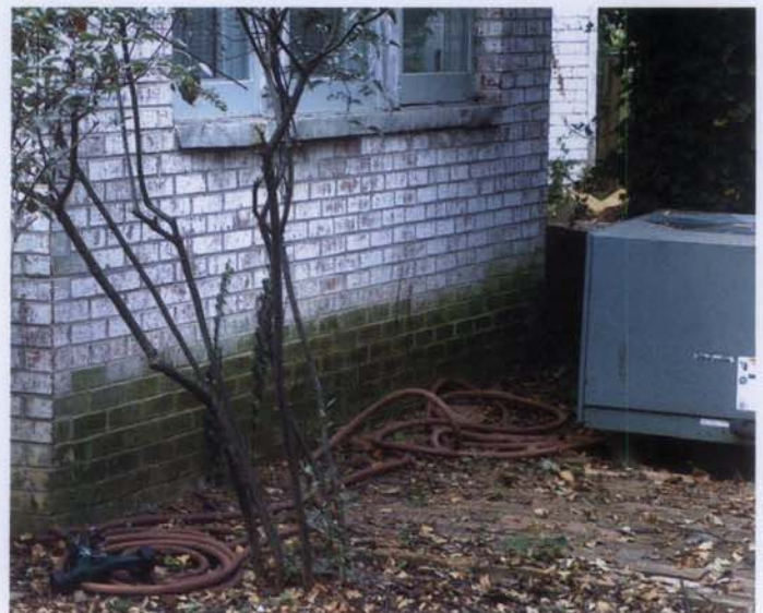
Figure 16. This chronically wet area has a mildew bloom brought on by heat generated from the air-conditioning condenser unit. The dampness could be caused by a clogged roof gutter, improper grading, or a leaking hose bibb.
