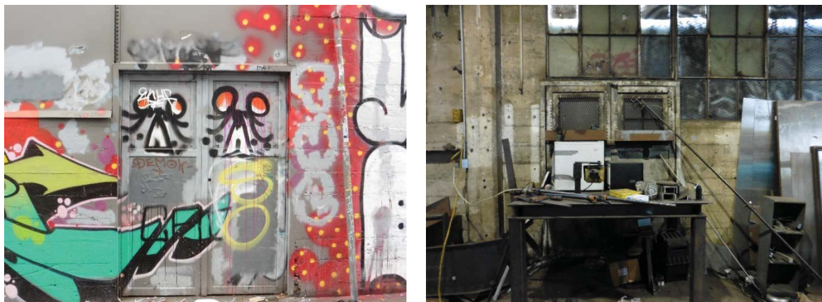
Figure 6: Exterior (left) and interior (right) views of the Berwick Place façade pedestrian doors.
