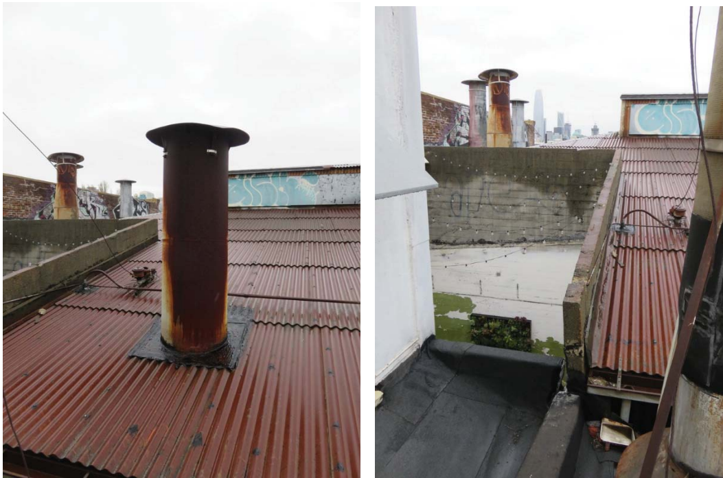
Above left: view of chimneys at rear of building and miscellaneous attachments at roof and parapet wall. Above right: additional view at rear of building; note that parapet wall has spall at top and appears to be leaning out slightly (ARG, 2018).
