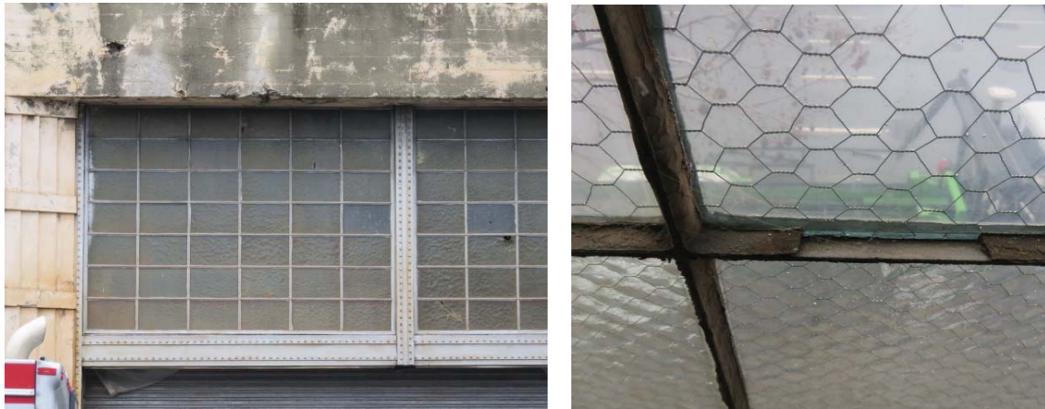
Above left: view of storefront assembly at west side of Harrison Street façade, including riveted frame and steel windows with textured wire glazing. Above right: detail view of missing glazing putty at Harrison Street window interior (ARG, 2018).
