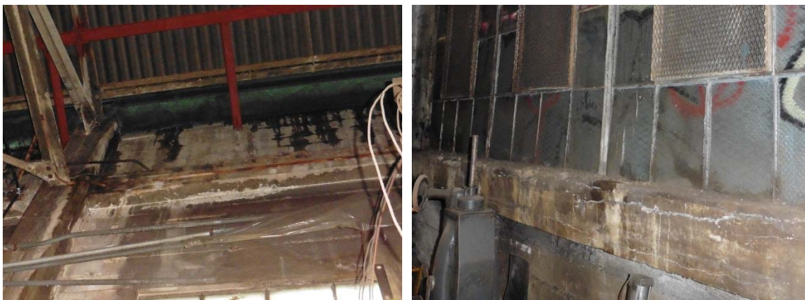
Figure 17: (Left) Water penetration and associated efflorescence at the roof line on the interior of the concrete wall at the Berwick Place façade; (Right) Horizontal cracking through the interior window sills at the Berwick Place façade.
