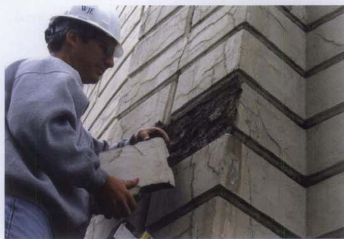
Figures 14. Layers of architectural concrete that have debonded (spalled) from the surface were removed from a historic water tank during the investigation performed to assess existing conditions. Photos: Anita Washko, Wiss, Janney, Elstner Associates, Inc.
