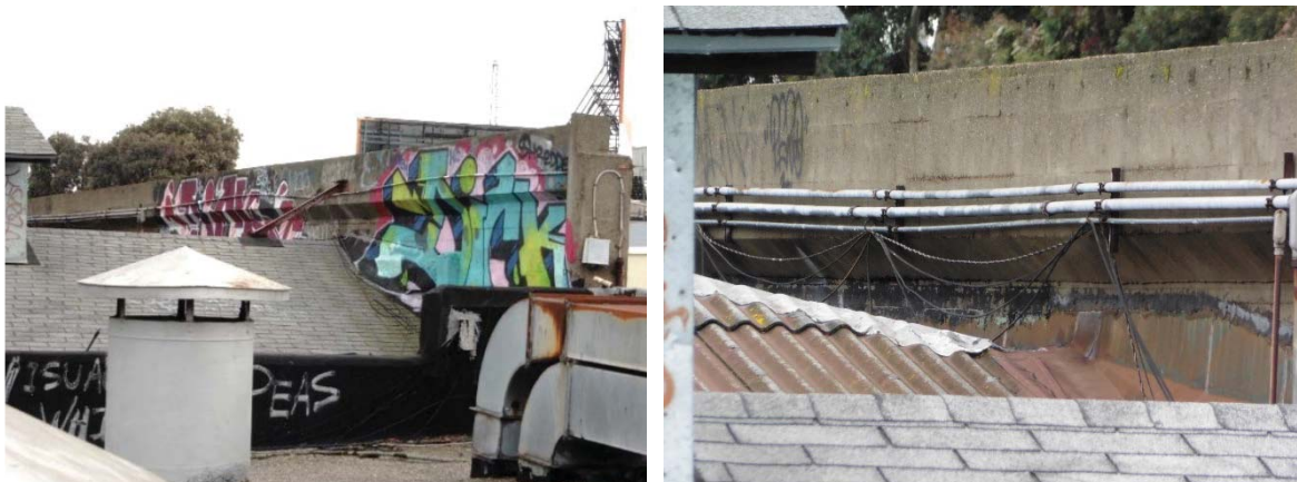
Figure 10: (Left) The west end of the rear side of the Harrison Street concrete parapet with asphalt shingle covered west roof and monitor (neighboring building in foreground); (Right) Close-up view of the parapet wall above a section of the east roof.
