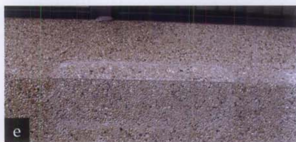
Figure 18. (a) Exposed aggregate precast concrete is sounded with a hammer to detect areas of deterioration. Corrosion of the exposed reinforcing steel bar has led to spalling of the adjacent concrete. (b) Samples of aggregate considered for use in repair concrete are compared to the original concrete materials in terms of size, color, texture, and reflectance. (c) Various sample panels are made using the selected concrete repair mix design for comparison to the original concrete on the building, and the mix design is adjusted based on review of the samples. (d) After removal of the spall, the concrete surface is prepared for installation of a formed patch. (e) Prior to placement of the concrete, a retarding agent is brush-applied to the inside face of the formwork to slow curing at the surface. After the concrete is partially cured, the forms are removed and the surface of the concrete is rubbed to remove some of the paste and expose the aggregate to match the original concrete.
