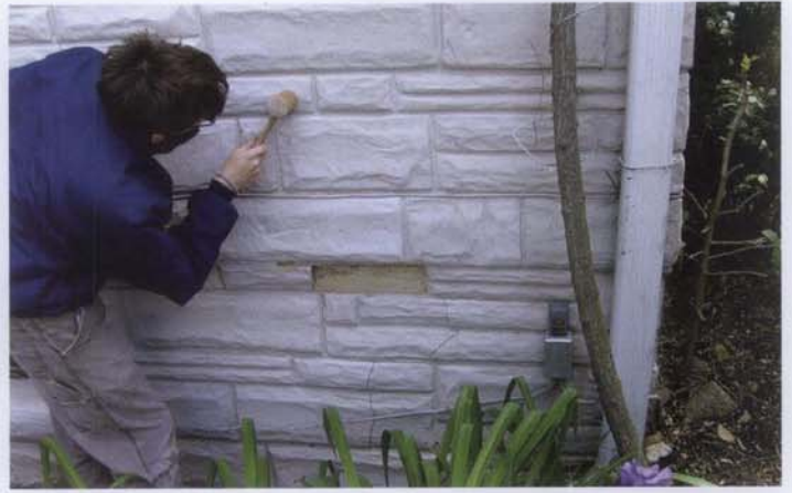
Figure 6. Stucco applied to an exterior wall or foundation was intended to function as a watertight surface. Unless maintained, rainwater will penetrate open joints and cracks that may occur over time. A spalled section of stucco indicates some damage has occurred and a wooden mallet is being used to tap the surface to determine whether the immediate stucco has lost adhesion. Photo: Bryan Blundell.
