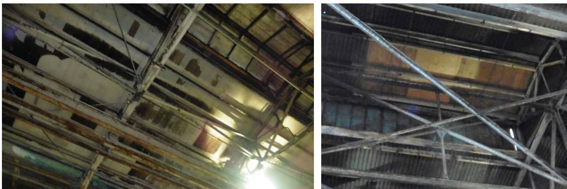
Figure 20: (Left) Wood sheathing on the ceiling of the west warehouse space; (Right) wood sheathing on the limited section of the east roof monitor where the corrugated metal has been replaced by asphalt shingles.
