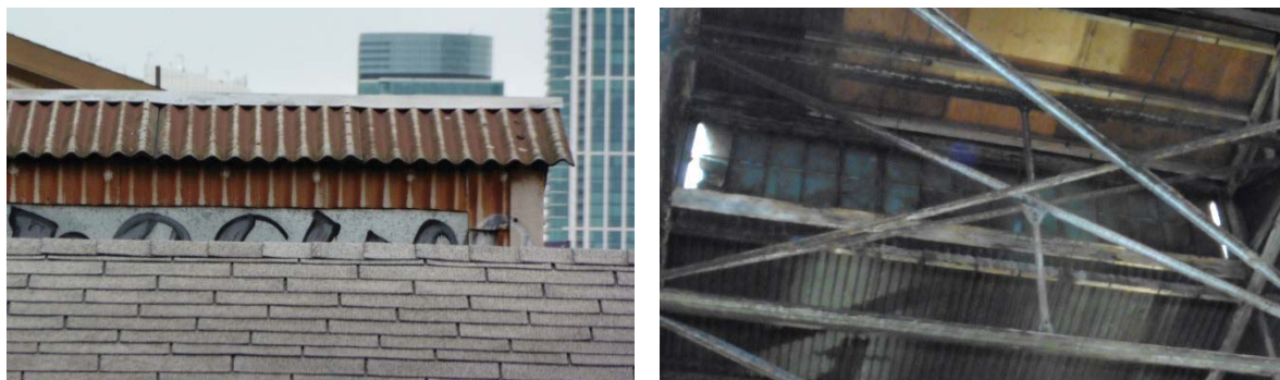
Figure 13: (Left) Boarded-up clerestory windows at east roof monitor; (Right) Existing boarded-up clerestory windows viewed from the east warehouse space.
