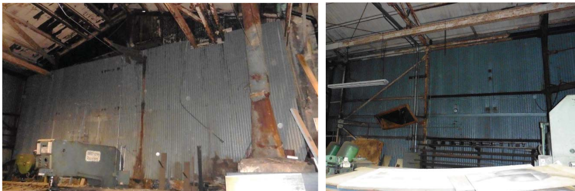
Figure 18: Corrugated metal on the rear (northwest) wall (left) and the side (southwest) wall (right) of the west warehouse space.
