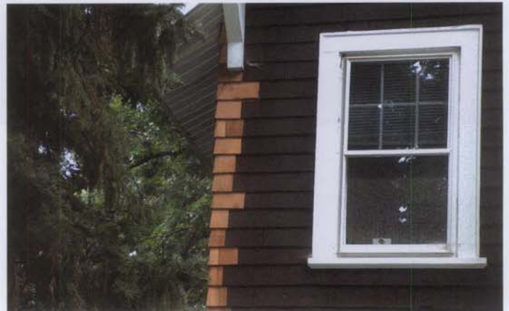
Figure 7. One of the advantages of wood shingles as a wall covering is that individual shingles that are damaged can easily be replaced. On this highly exposed corner, worn shingles have been selectively replaced to help safeguard against water damage. The new shingles will be stained to match the existing shingles.
