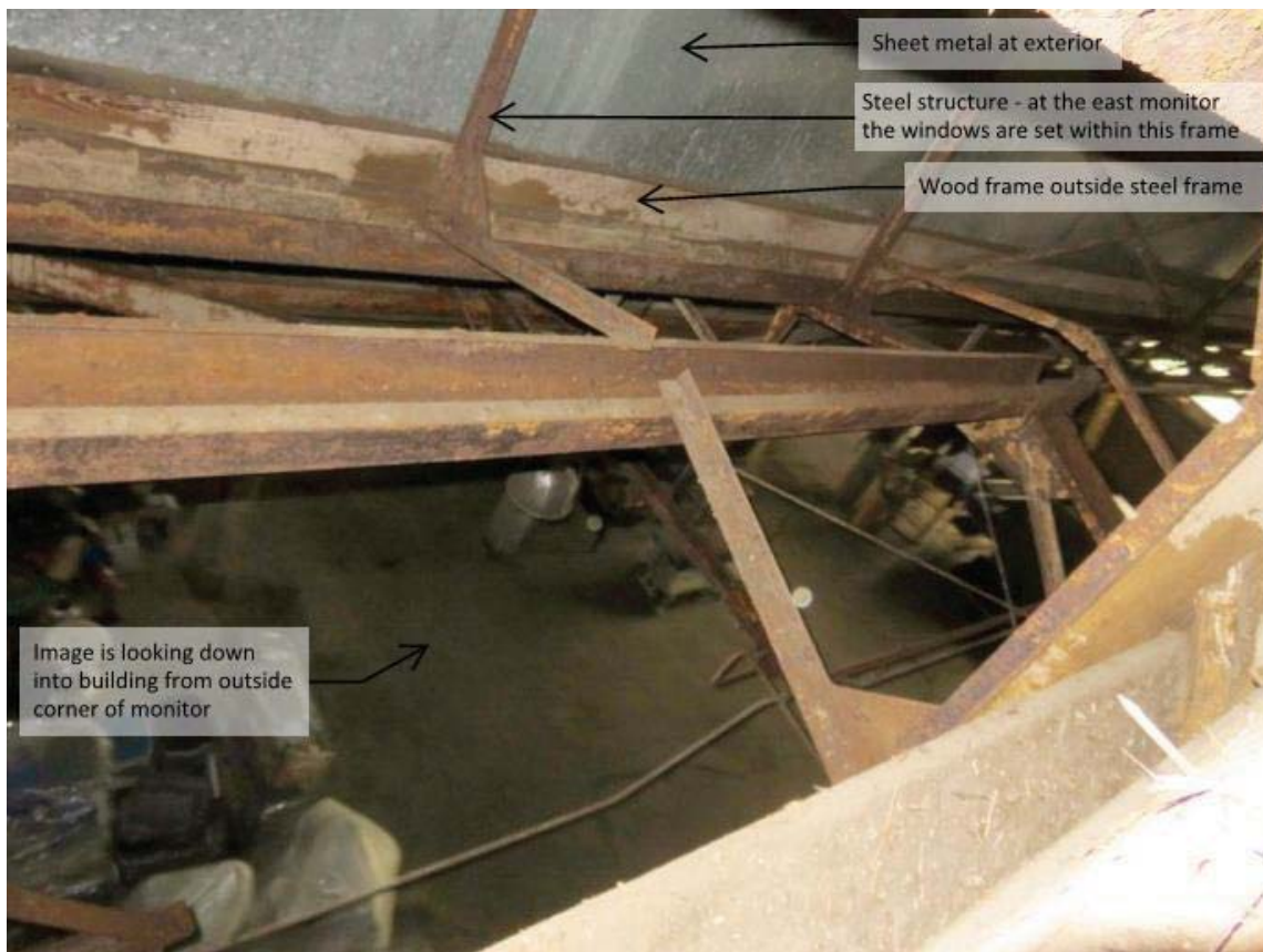
View from outside west monitor looking down into building. Note there is no evidence of previous window attachment at the steel frame (ARG, 2018, including annotation).
