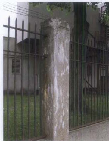
Figure 15. Evidence of moisture movement through concrete is apparent in the form of mineral deposits on the concrete surface. Cyclic freezing and thawing of entrapped moisture, and corrosion of embedded reinforcement, have also contributed to deterioration of the concrete column on this fence at Crocker Field in Fitchburg, Massachusetts, designed by the Olmsted Brothers.
