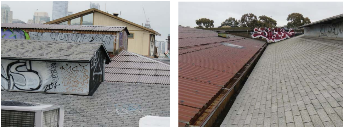
Above left: view looking east from neighboring building, showing both roof monitors, which have been enclosed with sheet metal. Above right: view looking south showing gutter between two roof sections and backside of Harrison Street parapet wall.
