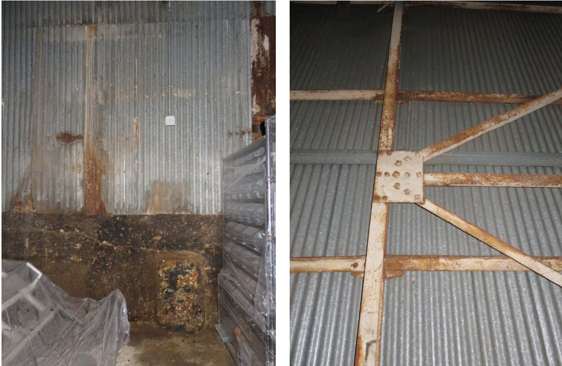
Above left interior wall at west side of building, including irregularly corroded corrugated metal paneling above a heavily stained concrete wall. Above right: typical surface corrosion at interior steel framing (ARG, 2018).
