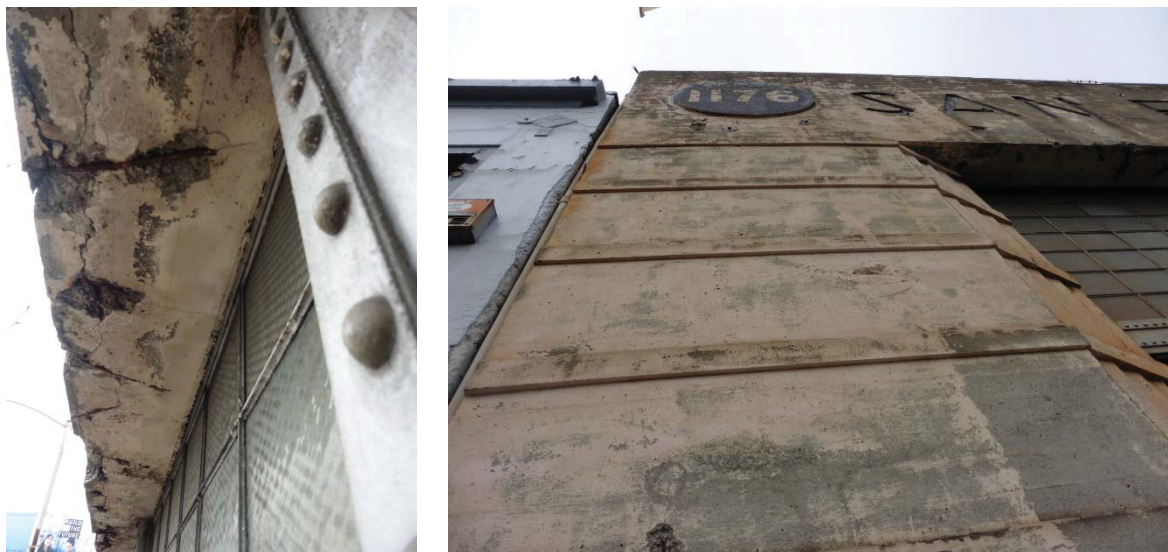
Figure 2: (Left) Spalled concrete above wall, window & door assembly is in poor condition; (Right) Concrete at the west end of the Harrison Street façade is in fair condition.
