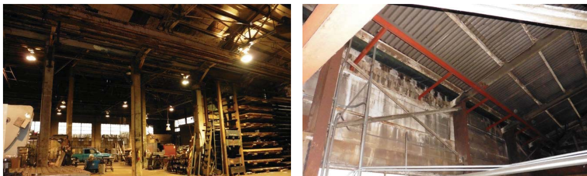
Figure 19: (Left) View into the east warehouse space from the west warehouse space showing the exposed rafters, trusses and purlins, and the concrete-covered structural steel columns; (Right) Structural ties (red) added to the Harrison Street façade concrete wall.
