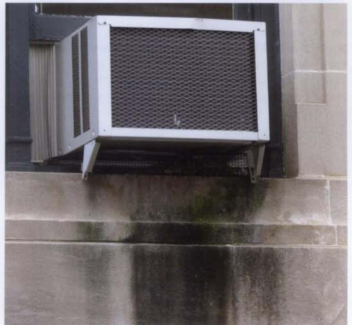
Figure 13. Window air conditioning units can cause damage to surfaces below when condensation drips in an uncontrolled manner. Drip extension tubes can sometimes be added to direct the discharge.
