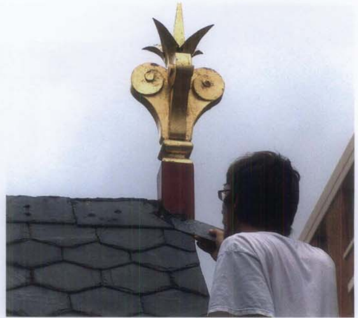
Figure 5. The use of a sealant to close an exposed joint is not always an effective long-term solution. Where this decorative wood element connects to the slate roof, the sealant has failed within a short time and a proper metal flashing collar is being fitted instead. Photo: Bryan Blundell.
