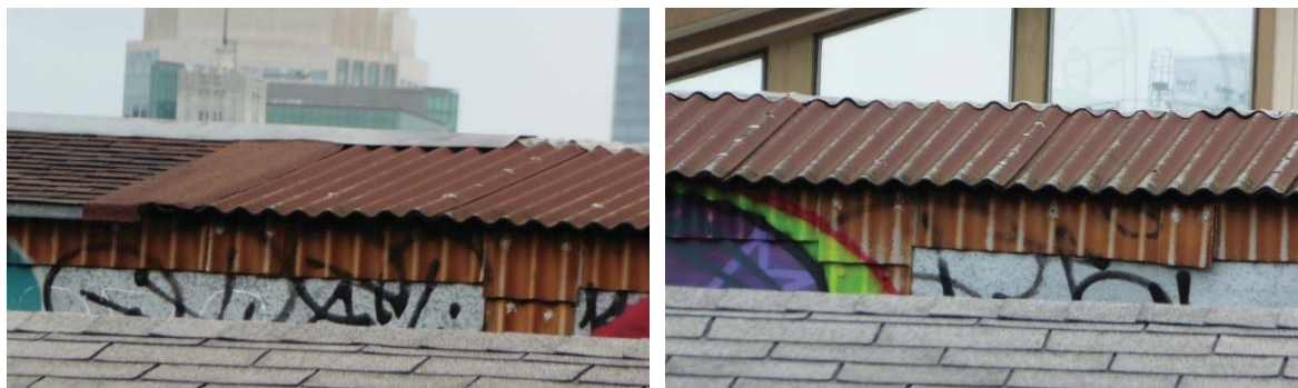
Figure 11: (Left) East roof monitor showing connection between corrugated metal and asphalt shingle roofing; (Right) Warping and gaps in the east roof monitor flashing and displacement of corrugated siding.
