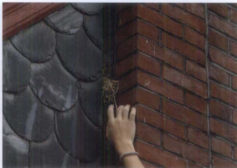
Figure 14. When inspecting connections between projections and the main building, look for areas where birds, bees and pests may enter or nest. Birds have been nesting in this porch roof and the area is being cleaned of their debris. Where an opening exists, it may be necessary to cover it with a trim piece, screening, or sealant. Photo: Bryan Blundell.
