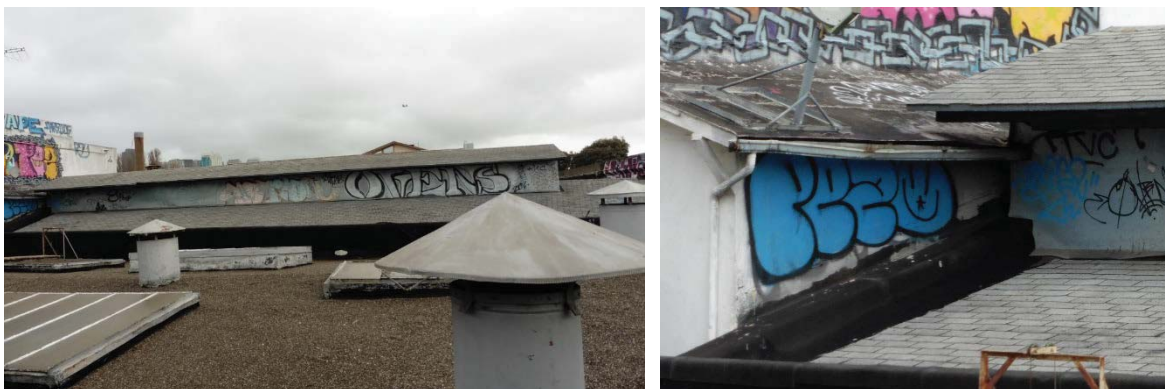
Figure 12: (Left) Asphalt shingle-covered west roof and monitor; (Right) Connection between neighboring pitched roof with damaged gutter adjacent to west roof.
