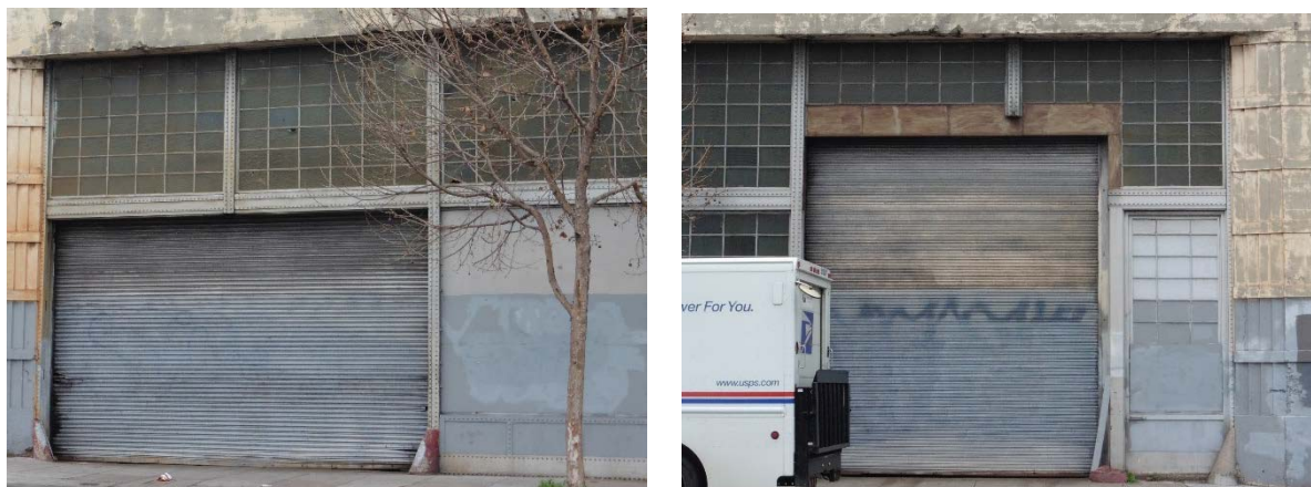
Figure 4: (Left) Wide metal roll-up door at west end of façade and (right) tall metal roll-up door at east end of façade inserted into the original wall, window, and door assembly.
