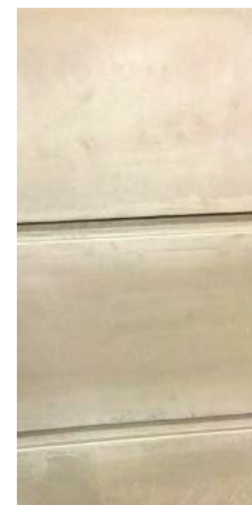
Stucco with Clear Coat Sealer
