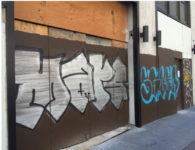
Boarded up storefronts on first story of primary facade.
