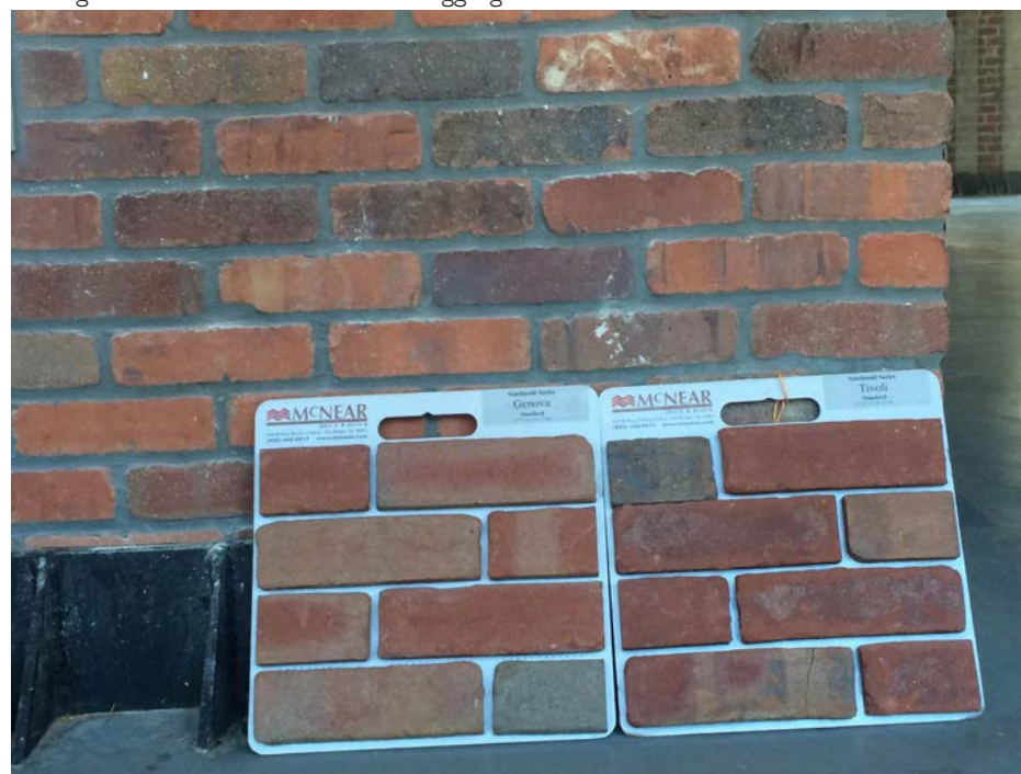
An existing door opening will be replaced with a window and the area below the new window will be infilled with veneer brick to match the adjacent brick veneer. Above photo shows two brick veneer colors being considered for the infill.
