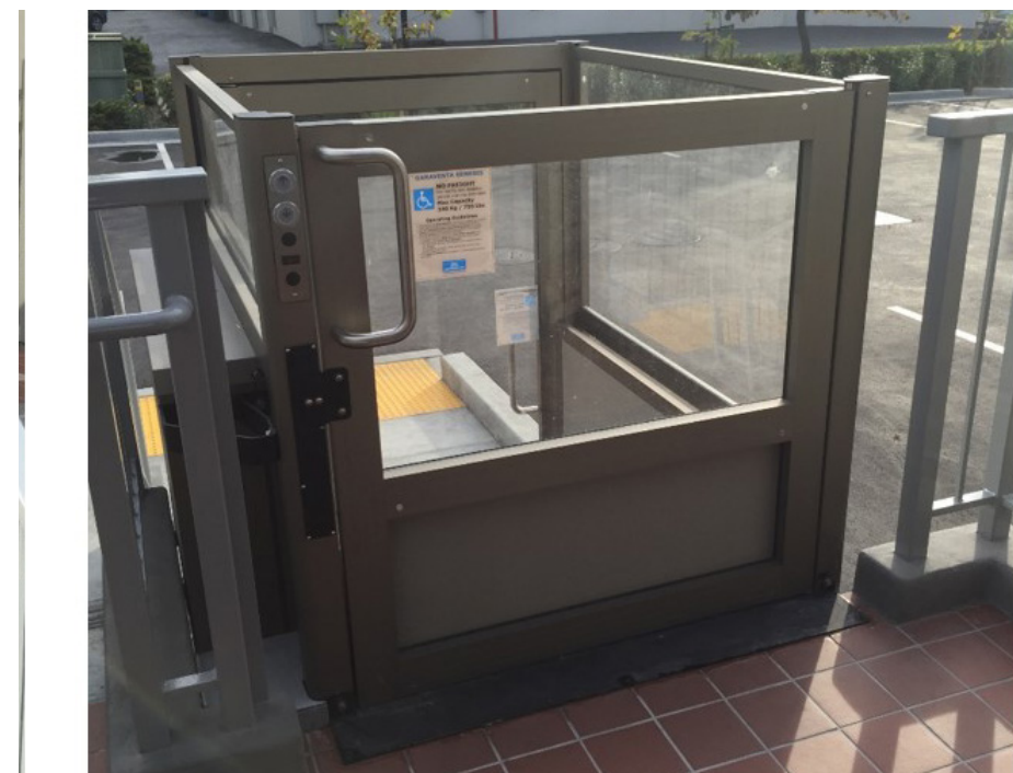
The proposed lift will be dark in color to complement the color palette of the railings.
