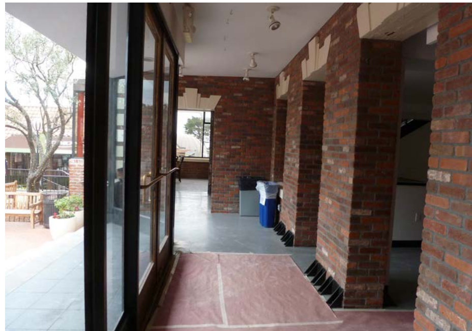
View of entry level of the west masonry facade, looking north. This portion of the wall is not original.
