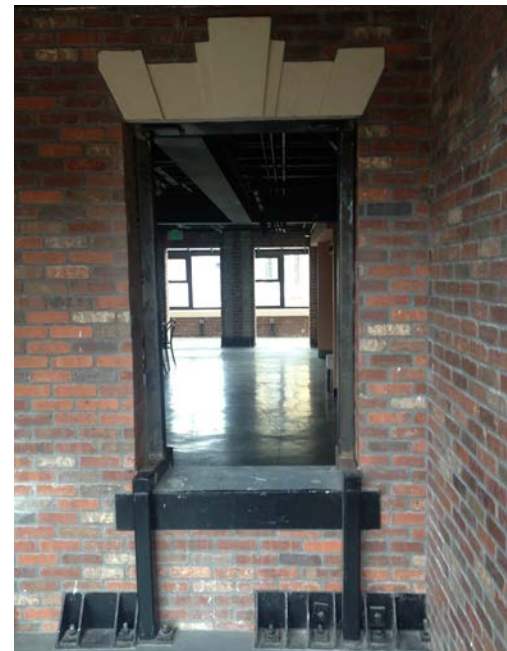
View of opening at west masonry facade. This portion of the wall is not original.
