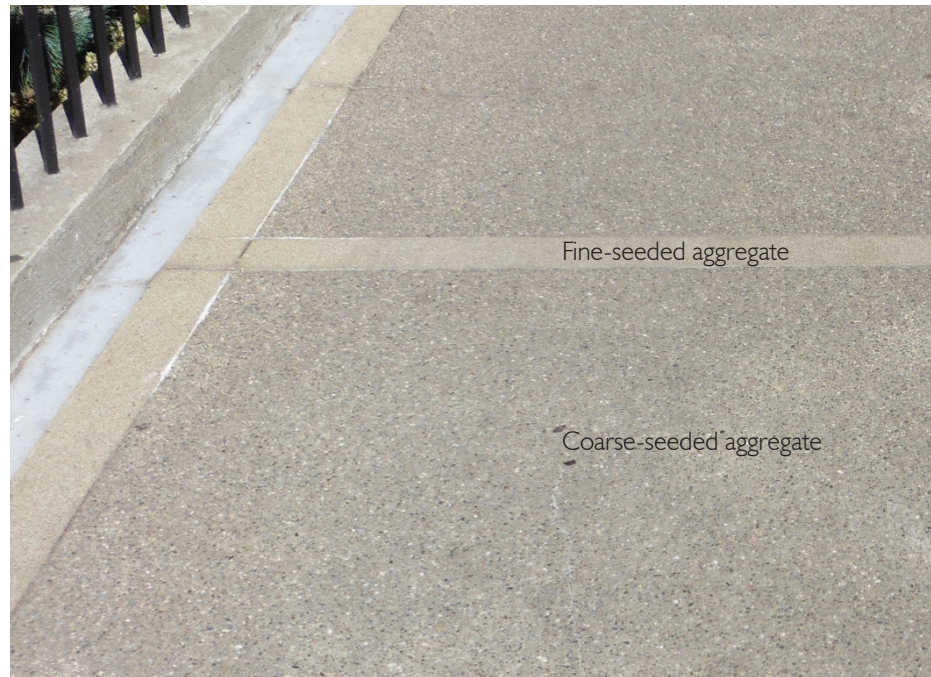
Original Halprin-era paving. The new steps will match the fine-seeded aggregate and the landing will match the coarse-seeded aggregate.
