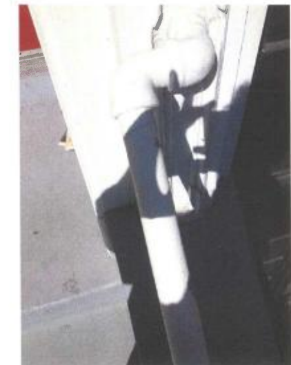
Existing railing to be replaced
