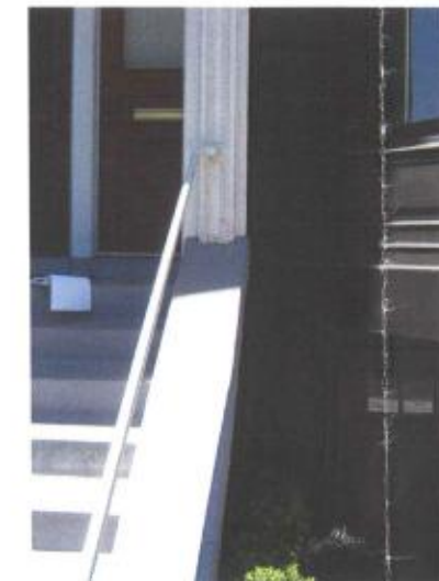
Existing railing to be replaced
