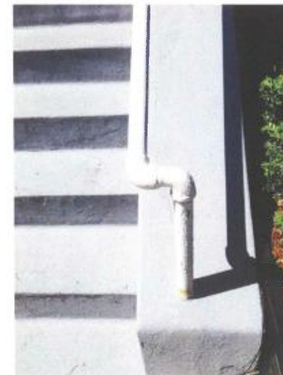
Existing railing to be replaced
