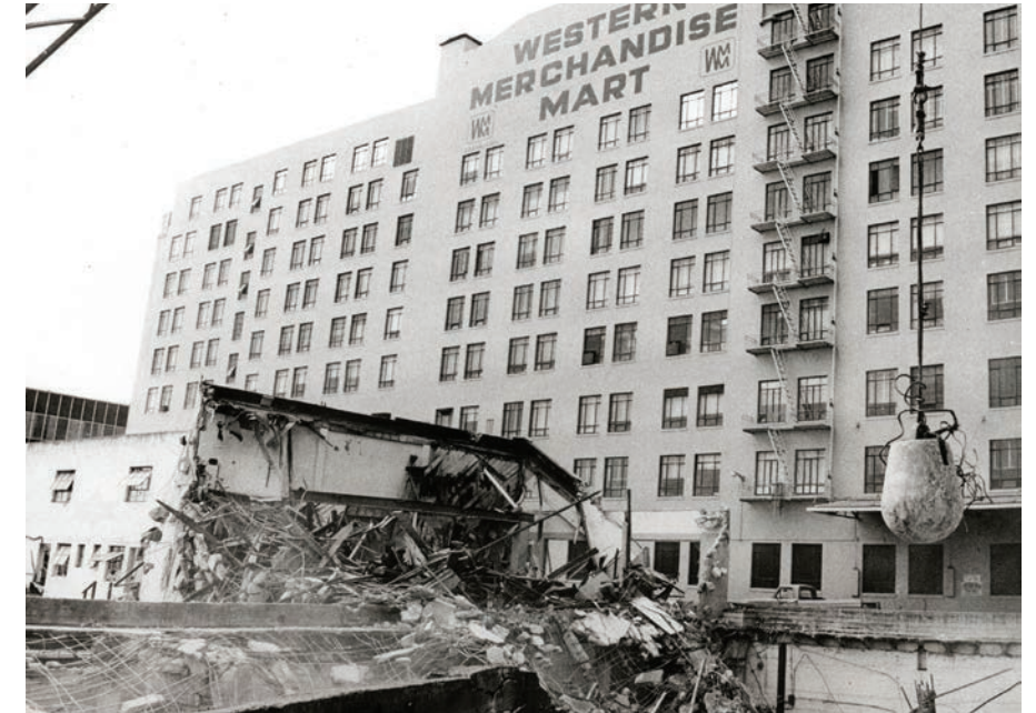
Demolition in preparation for Mart 2 construction with view of Stevenson Street facade, 1973 (Market Square Archives)
