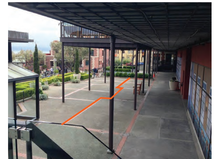
Paving from 1984 alterations. Note irregularity of grid.
