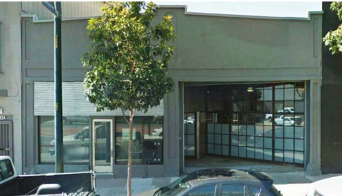
2620 3rd Street also with metal cornice detail and large ground floor entries
