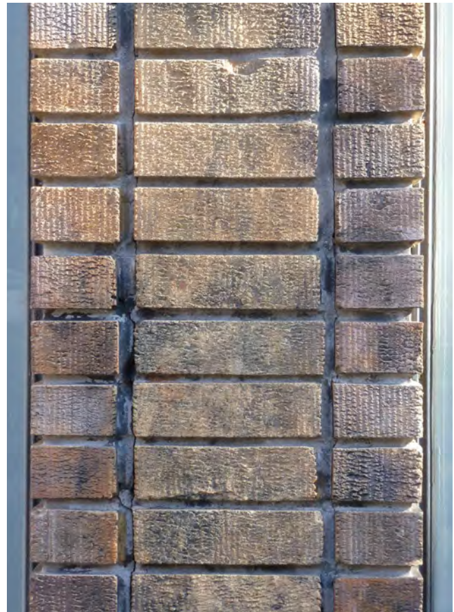
Figure 1. Typical brick pier; note mortar coloring and condition; deep recessed joint to be maintained.
