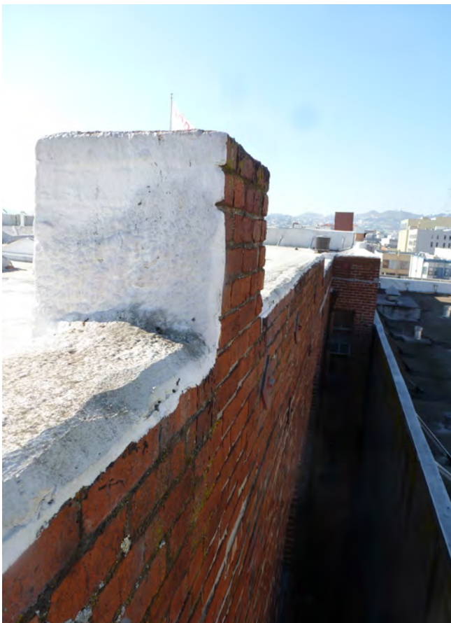
Figure 3. Unbraced ventilation stack at north wall.
