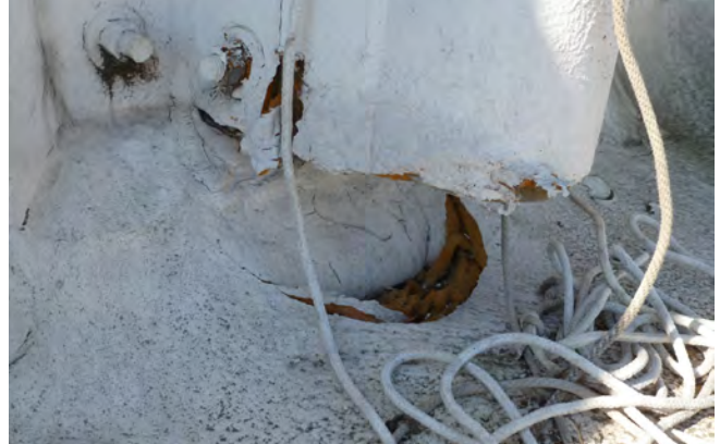
Figure 3. Detail of flagpole anchor; note corrosion and damage to roofing.
