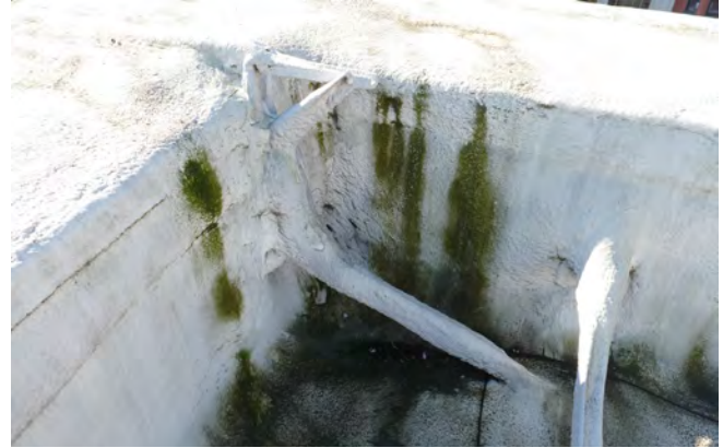
Figure 5. Bio-growth and water stains at roof. Investigate to if determine localized water damage exists.
