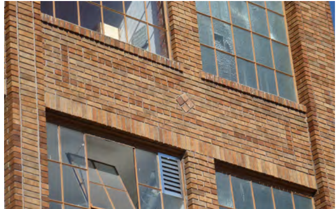
Figure 3. South elevation; note recessed mortar joints to be maintained and replicated in re-pointing.
