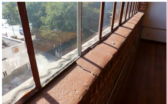
Figure 2: Concrete parge at south window sills, typical. Note level of localized cracking.
