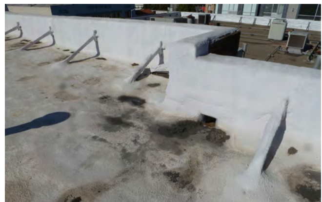
Figure 2. Roof at drainage opening in parapet; note parapet bracing and conditions near opening.
