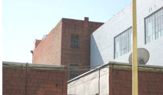
View south from Minna Street showing exposed portion of the north façade. (Page & Turnbull, April 2013)
