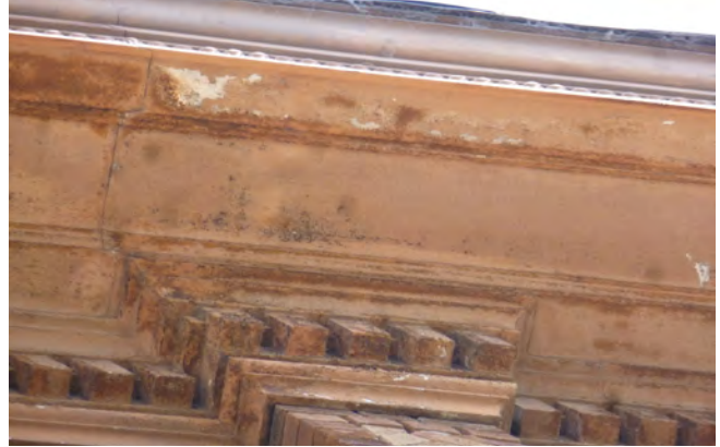
Figure 4. Cornice; conditions noted as typical.
