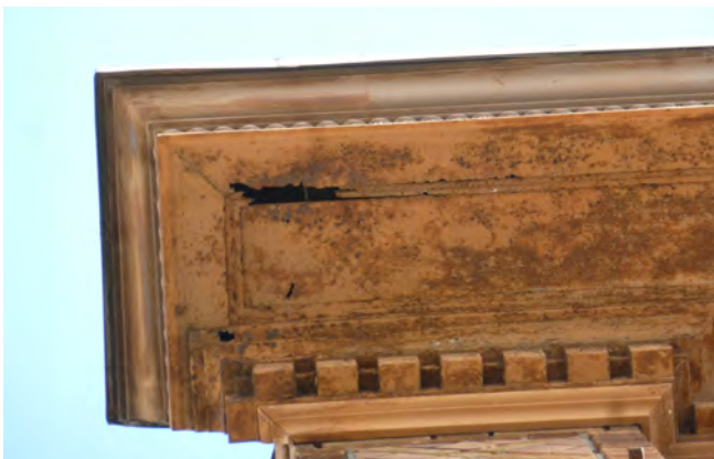
Figure 3. Cornice at northwest corner; localized areas of severe damage observed & requiring immediate repair.
