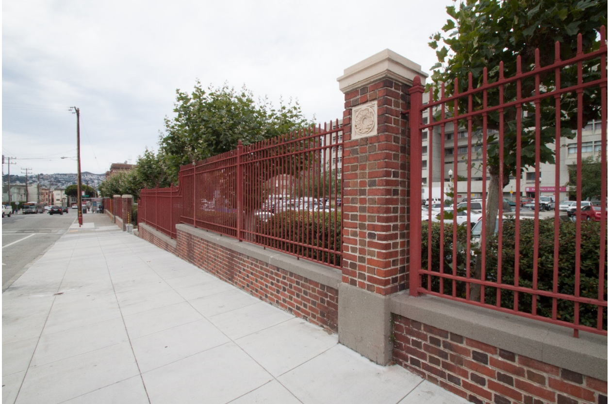
Figure 7. View of historic fencing that extends along southern edge of B/C lot, looking west (Architectural Resources Group, August 4, 2015).
