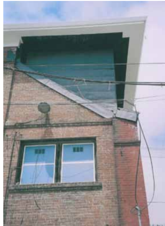
13. Office Building east elevation view of 2nd floor wall reconstruction at 1906 earthquake damage
