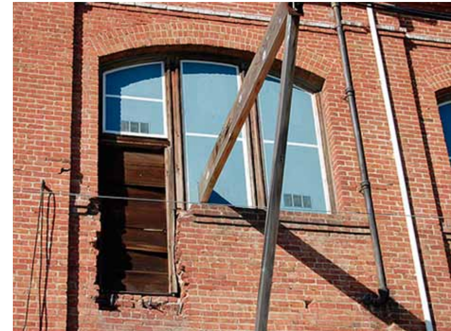
22. Office Building east elevation view of window modified into door opening in Carmen Strike of 1917
