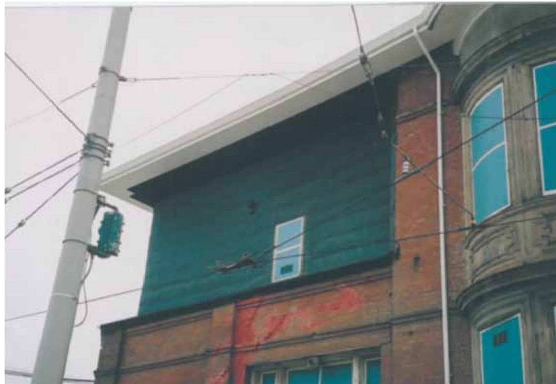
14. Office Building north elevation view of 2nd floor wall reconstruction at 1906 earthquake damage
