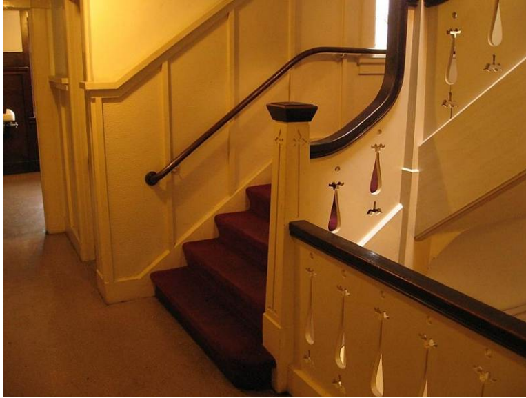
Detail of stairs at second floor as they rise toward the mezzanine.
