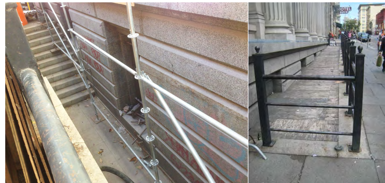
Figure 11: The light well is accessed by a stair that is located just to the north of the Entry Rotunda stair along Jones Street. The door to the basement is to the right of this photo. The floor to the right of the window opening is to be lowered to align with basement floor.
