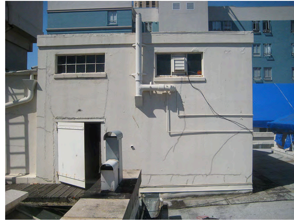
Figure 22: From the vent stack to the left is the area of the new East Hall that was approved in the earlier Certificate of Appropriateness. The window to the right is the one noted here.
