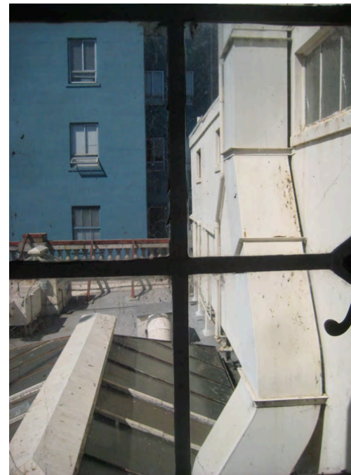
Figure 23: Looking west from the Penthouse Room. The three windows include the one in the upper right of the picture and the two beyond the duct near the center of the photo.
