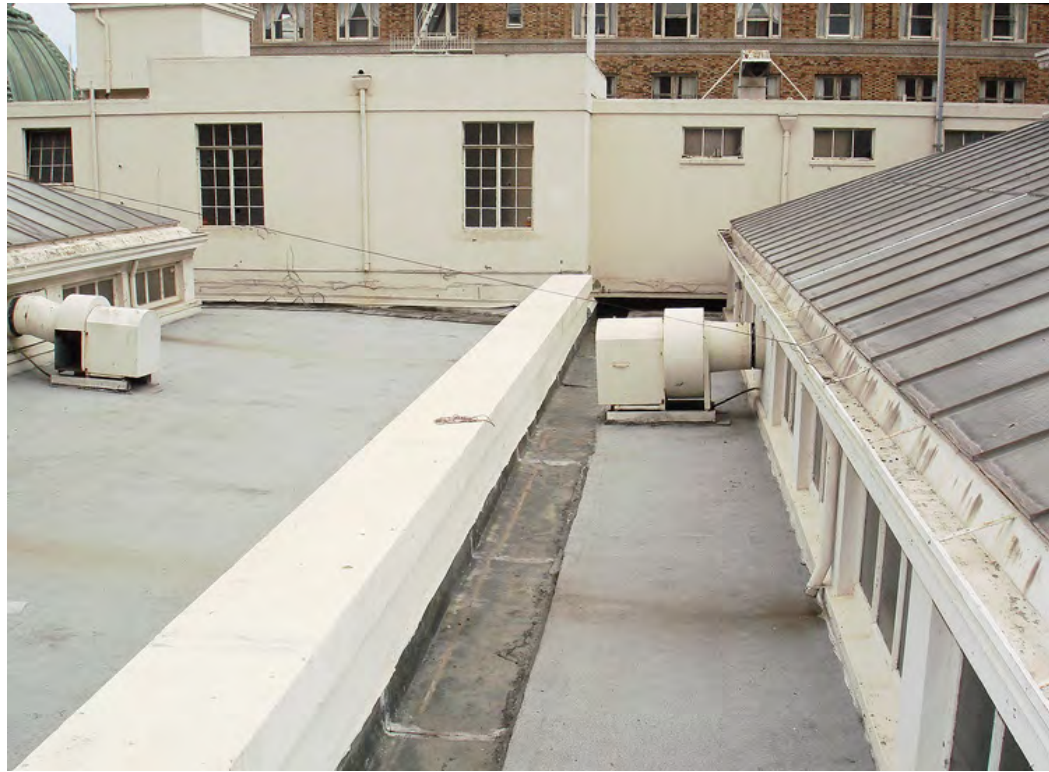
Figure 20: The tall window on the right (center of photo) becomes an exit door from the Penthouse Room as previously approved. The window on the left is proposed to be extended to the floor.
