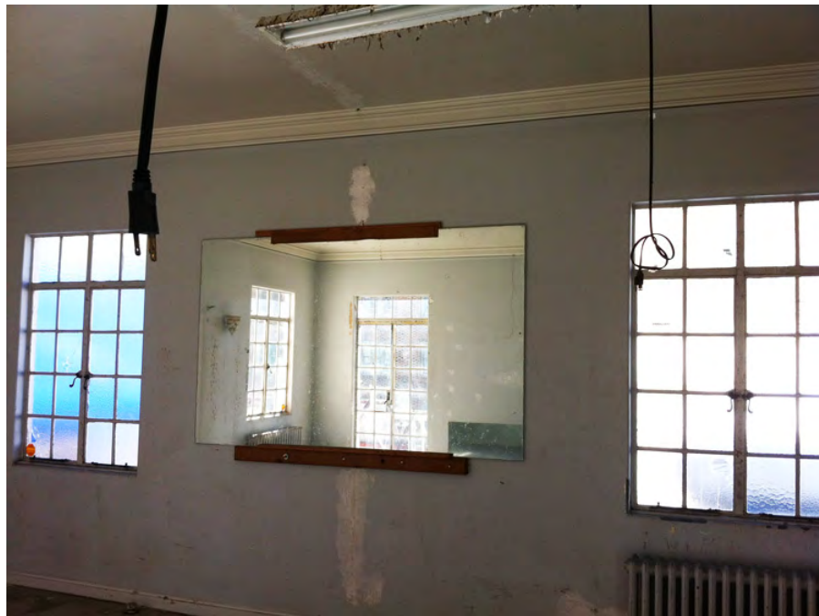
Figure 21: Interior of the Penthouse Room looking North. The window on the left will become an exit door that matches the two doors on the South wall that lead to the exterior roof deck. The window on the right is to be replaced with a fixed window proposed to match the exit door.
