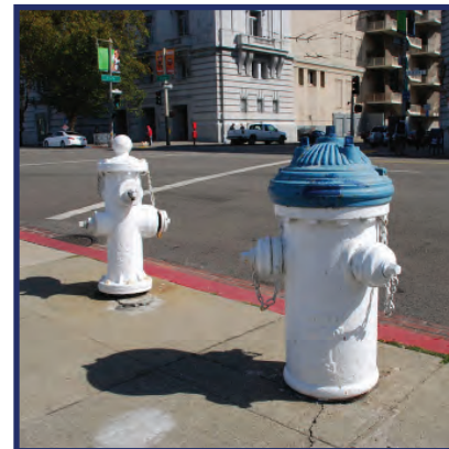
Low pressure fire hydrant and high pressure auxiliary water supply hydrant at Grove St
