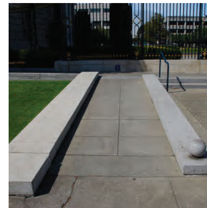
Accessible ramp to Opera House and Memorial Court with granite curbs at Van Ness Ave
