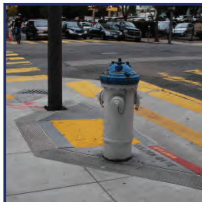
High pressure auxiliary water supply hydrant, Golden Gate Ave
