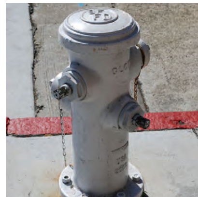
Low pressure hydrant along Franklin St
