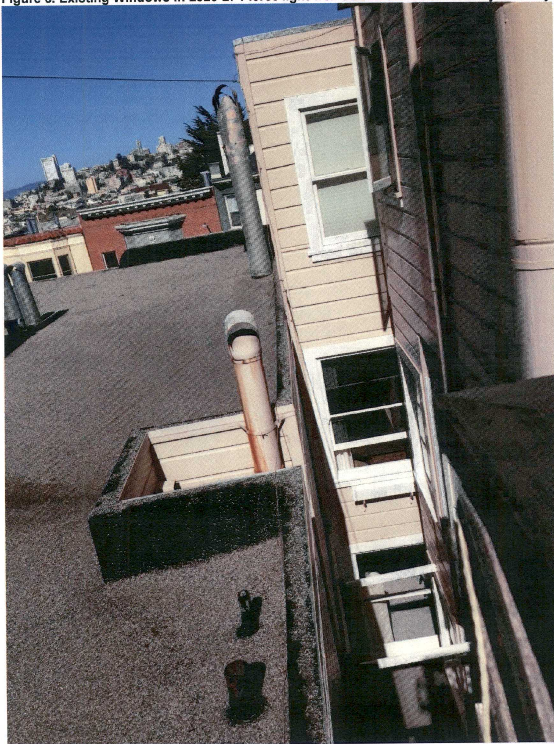
Figure 5. Existing Windows in 2823-27 Pierce light well that would be blocked by 4 th Story
