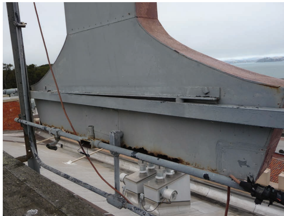
Photo of back side of the letter "i" showing corrosion at back face of letter.
