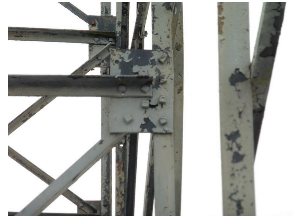
Photo of typical connections and members in the steel truss frame, showing corrosion and loss of paint
