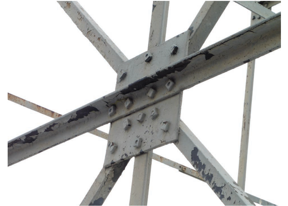
Photo of typical connection in the steel truss frame, showing corrosion and loss of paint
