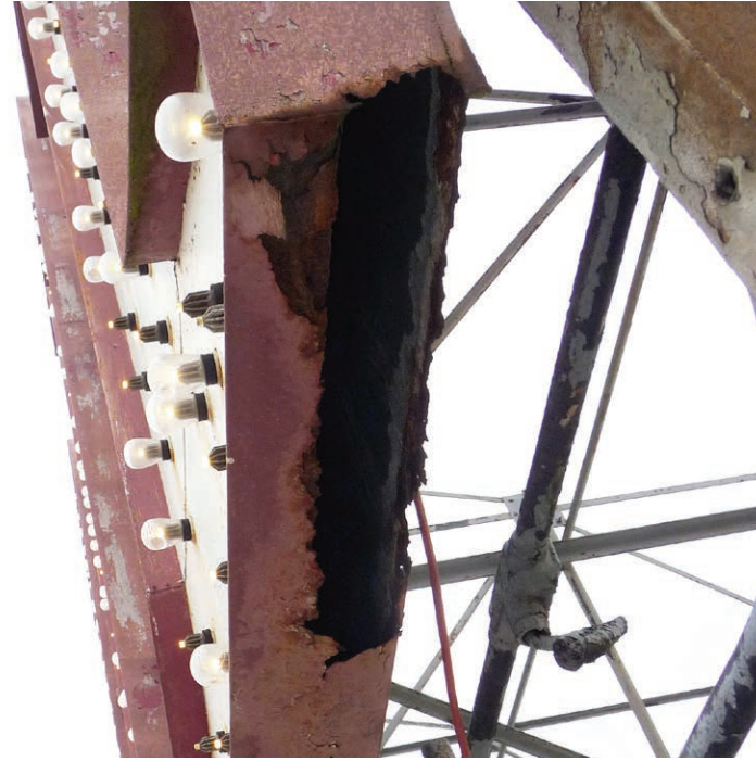
Close up of back side of letter showing corrosion at the bottom of the letter
