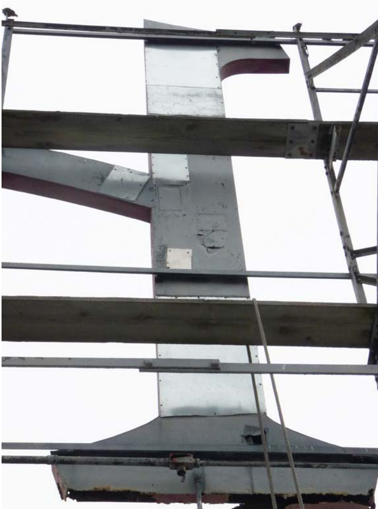
Figure 12 - Patches are visible at the back of the letters. The "h" letter exhibits the most patching, including open or edges of the patches which are open to the inside of the letter.
