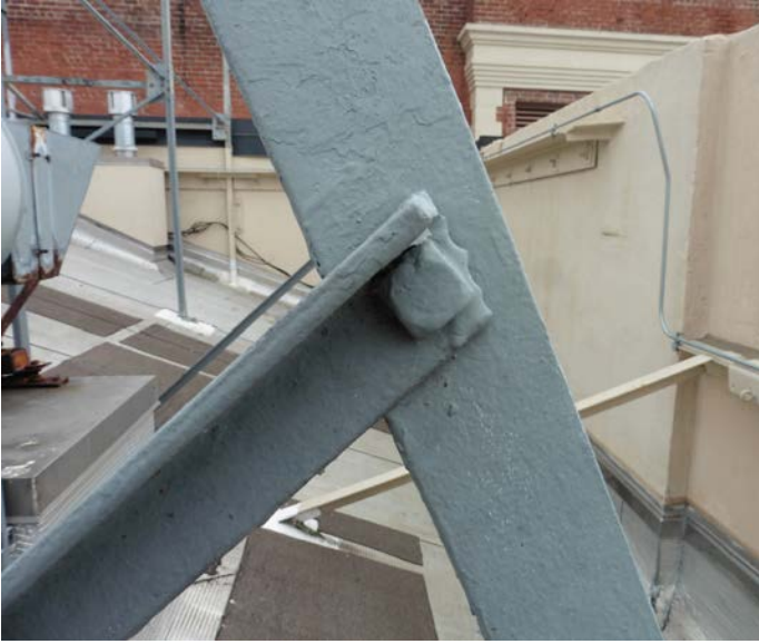
Figure 15 - A typical "good" condition connection of the armature, on the lower roof (Mustard Building), within easy arm's reach
