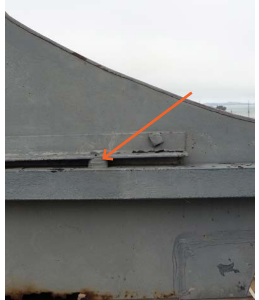
Figure 21 - Spacers are used between the angle to shim the letters into a level position.
