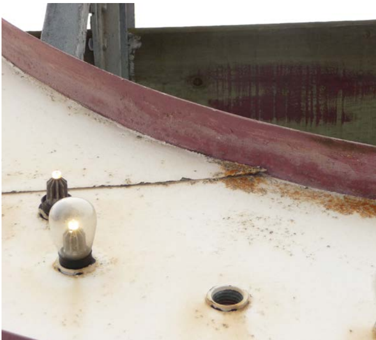
Figure 9 - Corrosion at the front face of this letter has resulted in the front piece of sheet steel pushing out. Note the various states of the lights: condensation within the globes, missing globes, or missing lights/lamps.
