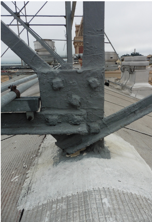
Figure 13 - Example of good condition connections at the roof, which have been waterproofed and painted more recently. These are common on the lower roof below the eastern half of "Ghirardelli"
