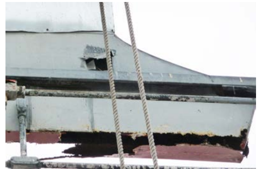
Figure 8 - Extensive deterioration at the base of a letter due to water intrusion and/or ponding. The base here has sheared away at its edges.
