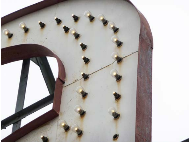
Figure 11 - The pieces of sheet steel that comprise the letters are separating or pulling away from each other at various joints, most typically where the face steel is pulling away from the sides or backing. Here the perimeter wall pieces become separated from where they previously have overlapped slightly.
