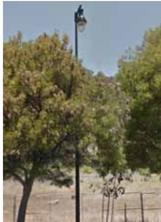
Existing Street Light Type 1
