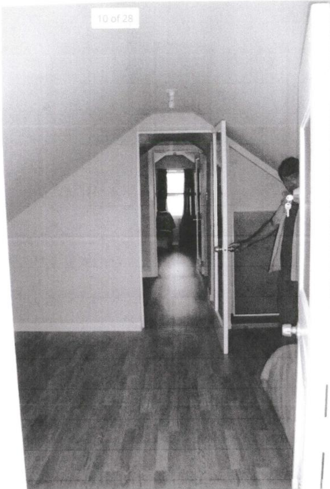
Photo of attic bedrooms; does not have required height for habitability
