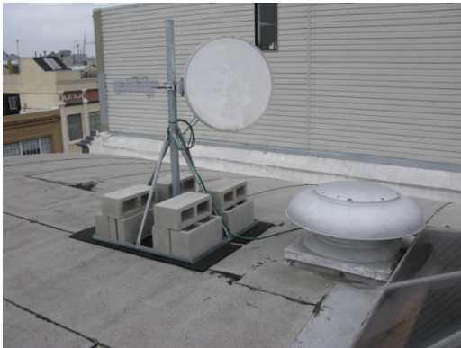
Miscellaneous roof equipment
