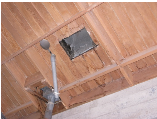
Moisture stains on board sheathing at penetration
