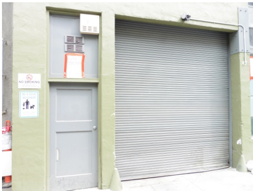
Original wood door to be replaced with metal; metal coiling door to be replaced with new storefront
