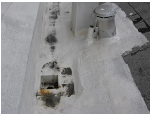
Missing drain cover
