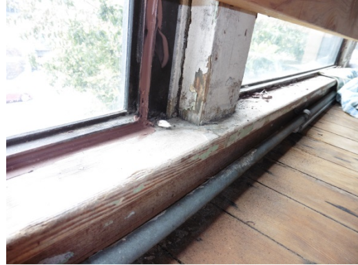
Water damaged wood sills and wood floor at Howard Street
