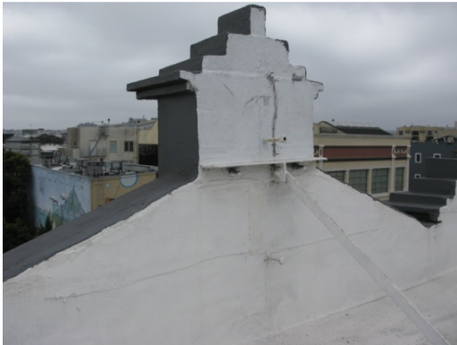
Crack at center parapet
