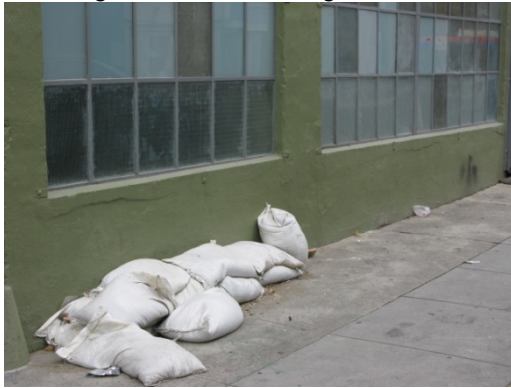
Portions of walls below windows have had prior repairs
