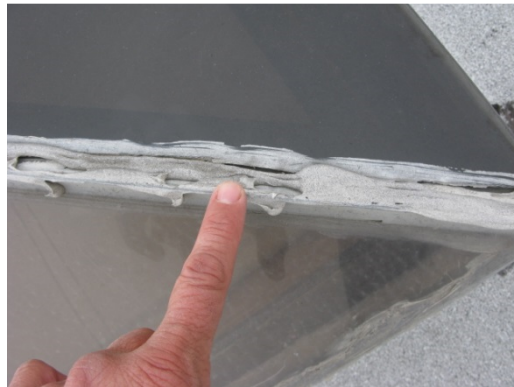
Openings in sealant joint at repaired skylight
