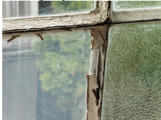
Typical failed glazing putty
